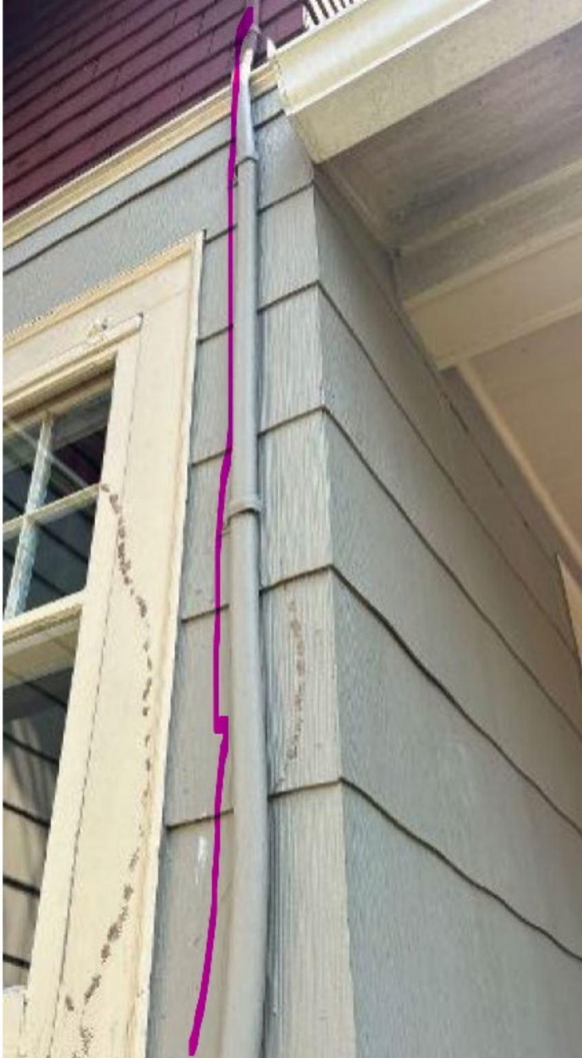
Utility Meter after Install
