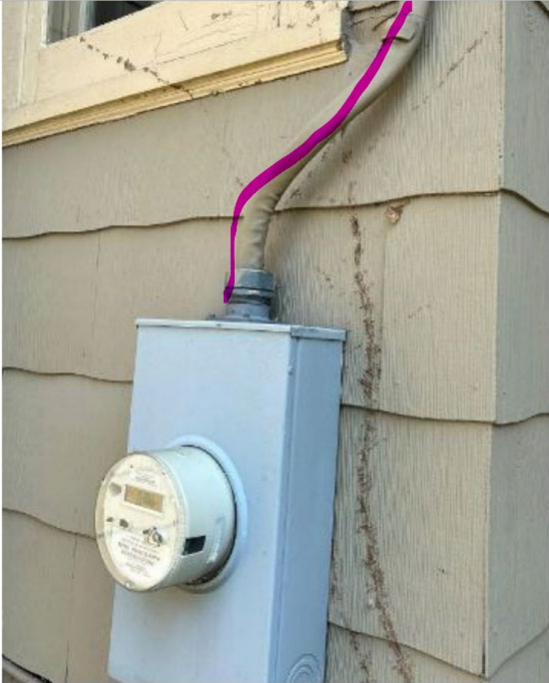
Utility Meter after Install
