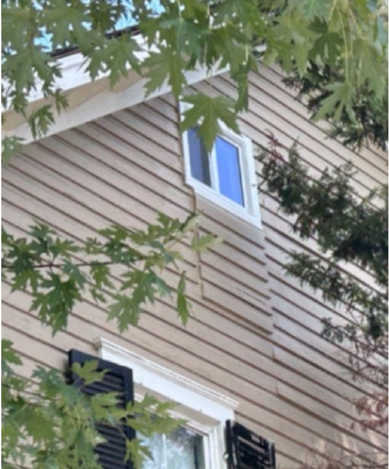
Figure 11: Closer exterior view of one of the altered windows showing details of the installation. Trim that matched the window below was also removed (September 2024, Historic Preservation Office).
