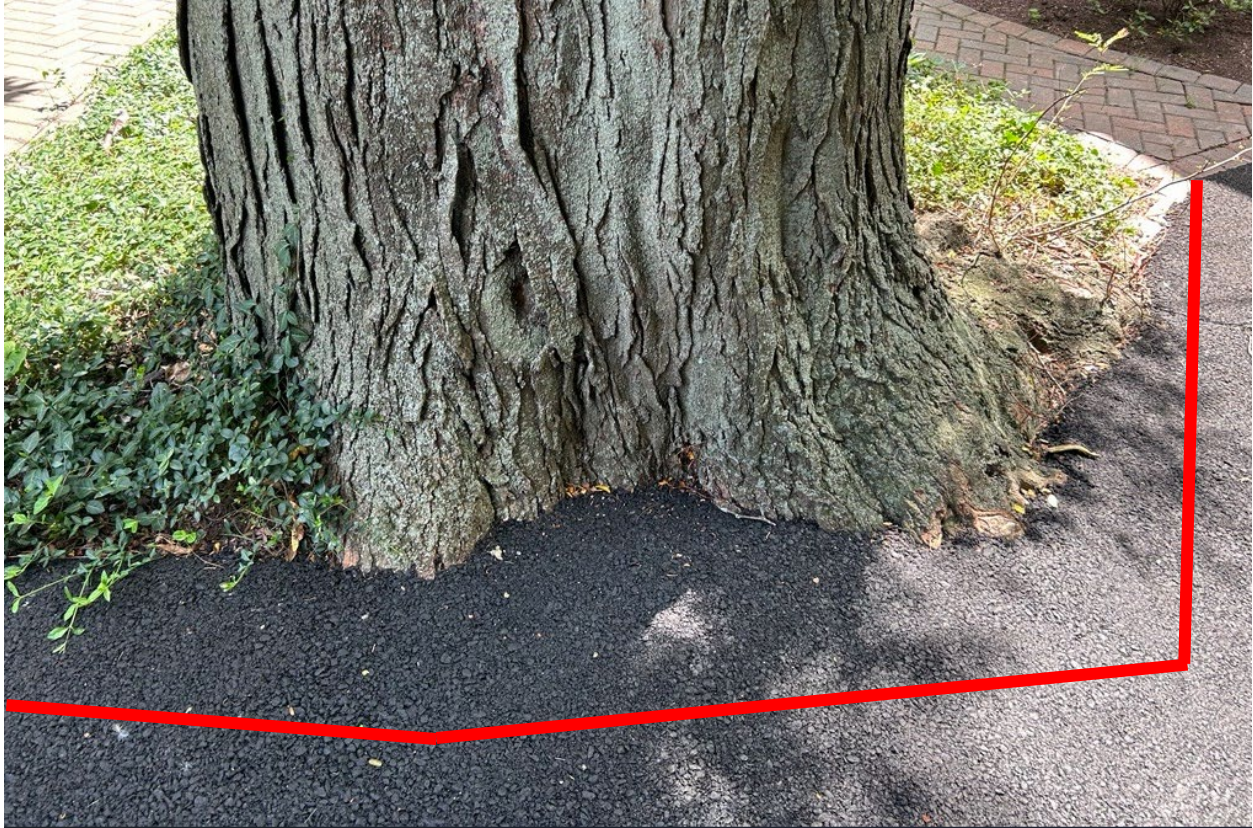
Figure 6: Asphalt paving was added up to trunk of the tree. Staff recommends the paving abutting the trunk be hand removed a minimum of 6 inches from the trunk, roughly beyond the red line marked above.
