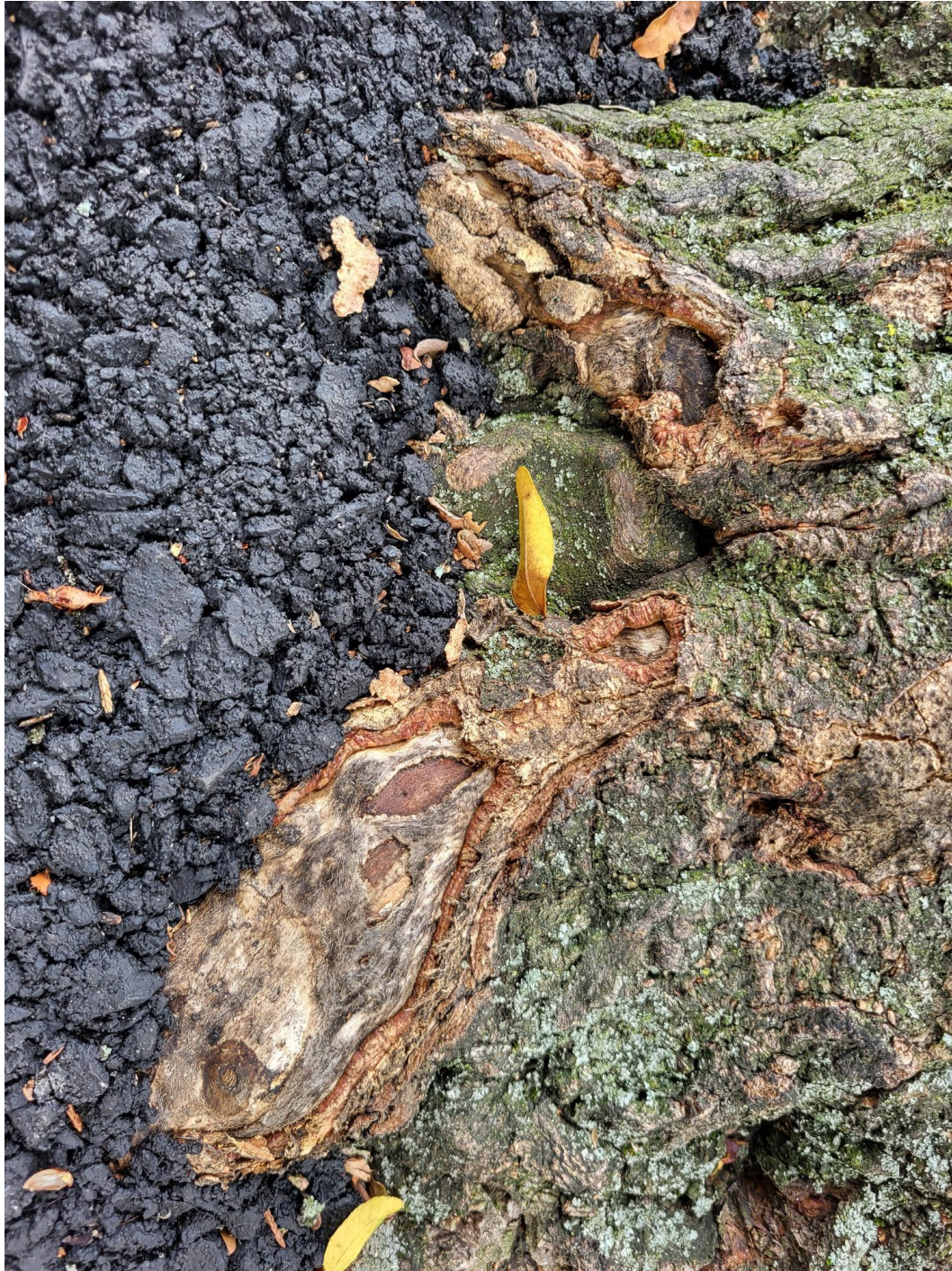
Figure 3: Base of tree showing driveway, and buttress root.
