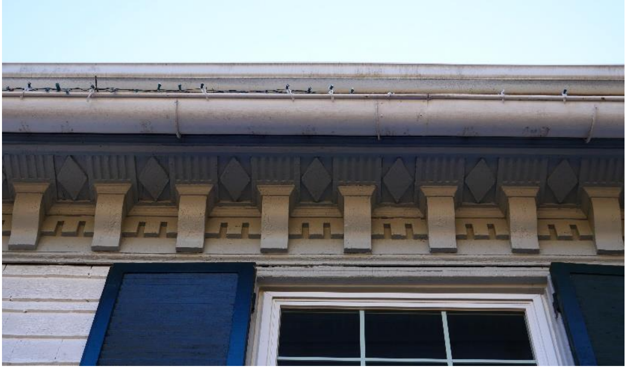
Figure 17: Detail view of the cornice on the 1901 dwelling, 2022. Source: Historic Preservation Office, Montgomery Planning.
