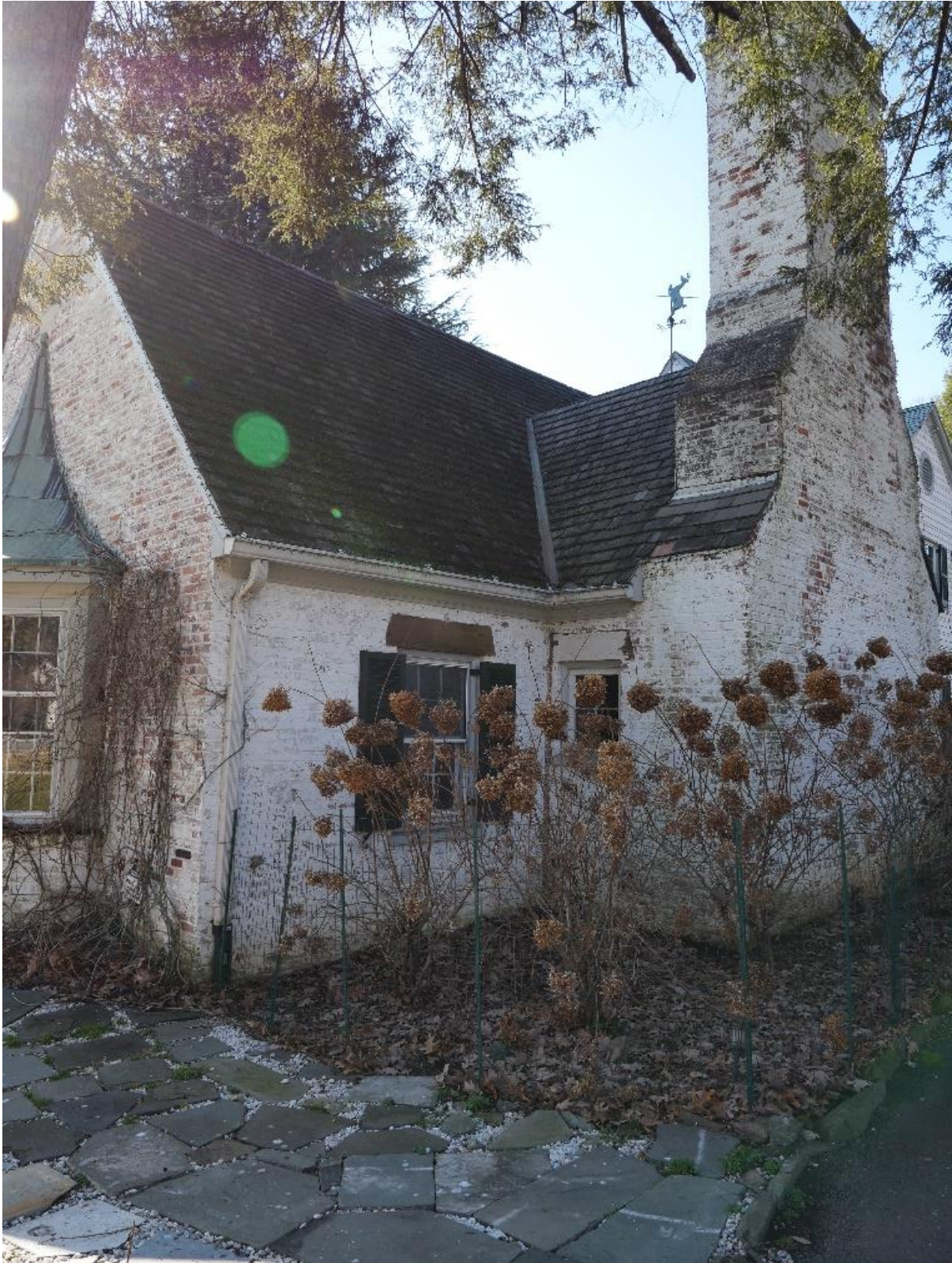
Figure 11: Axial view of the northeast elevation of the 1930 living room addition (looking southwest), 2022.
