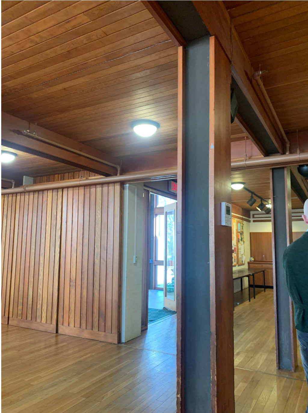
MD_Montgomery County_River Road Unitarian Church_0018 East interior wall of sanctuary beneath gallery showing wooden partition walls on left that slide along the track in the floor (Davenport January 2024)
