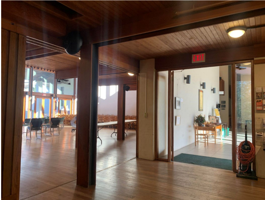
MD_Montgomery County_River Road Unitarian Church_0019 Northwest view from anteroom of sanctuary on left and entrance foyer on right (Davenport January 2024)
