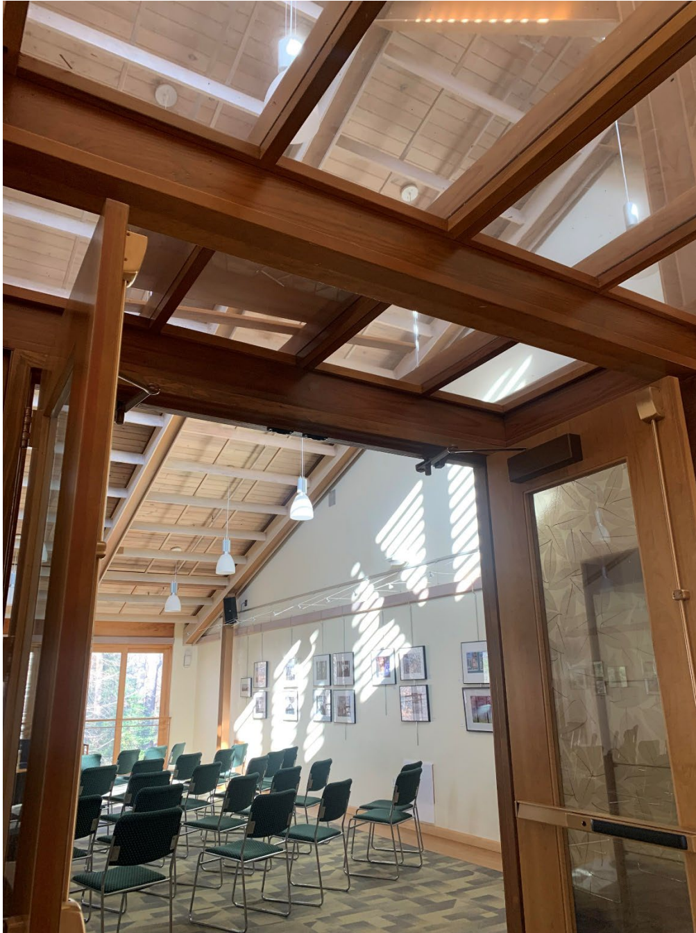
MD_Montgomery County_River Road Unitarian Church_0024 Northwest view of fellowship hall, interior of MFTA building (Davenport January 2024)
