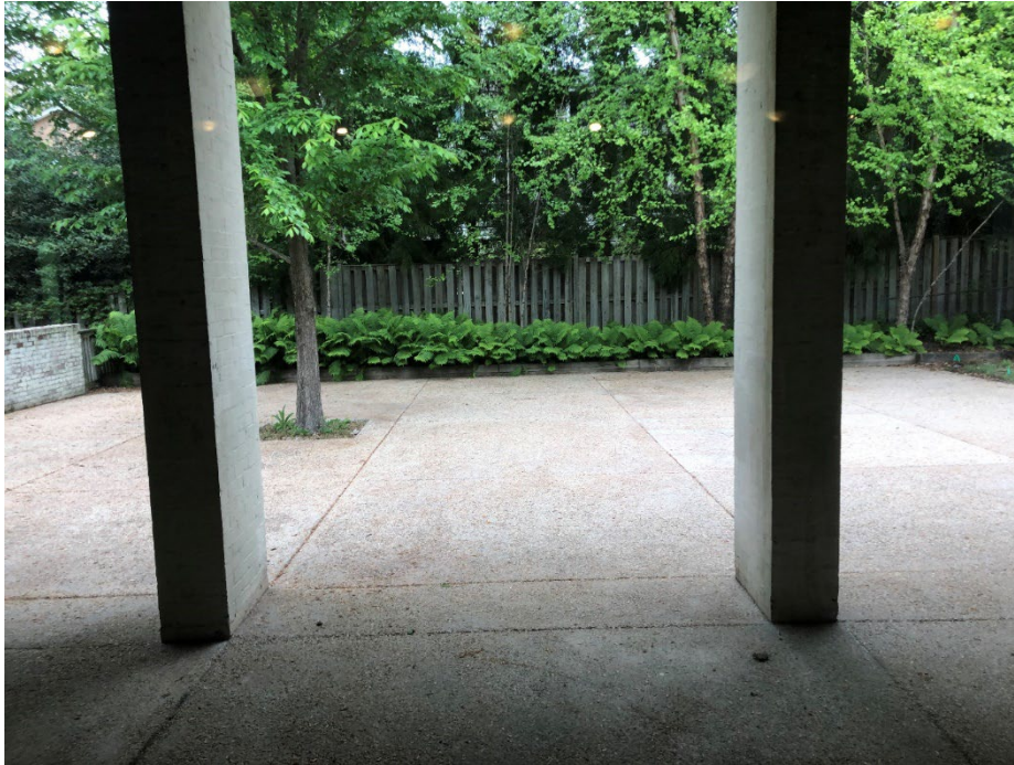
MD_Montgomery County_River Road Unitarian Church_0012 Patio on the north side of the classroom and office wing, view from interior hallway facing north (Hansman April 2024)
