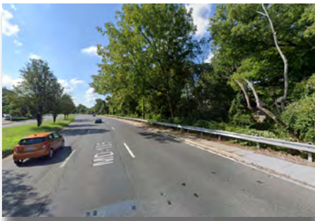
Guardrail behind sidewalk along Connecticut Avenue in Aspen Hill Photo Credit: Google Maps
