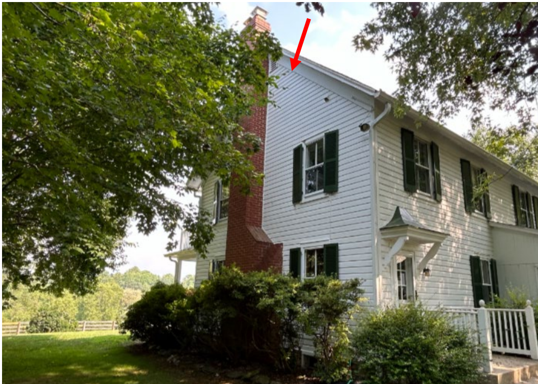
Figure 11: North elevation. The red arrow points to the location of the proposed casement window.
