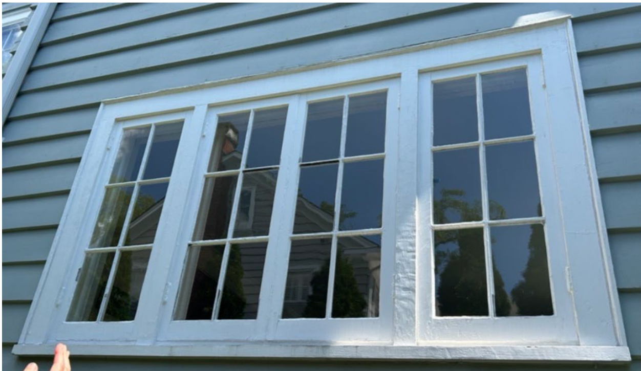
Figure 6: Detail of the four casement windows to be replaced with fixed windows of matching design on the west elevation.
