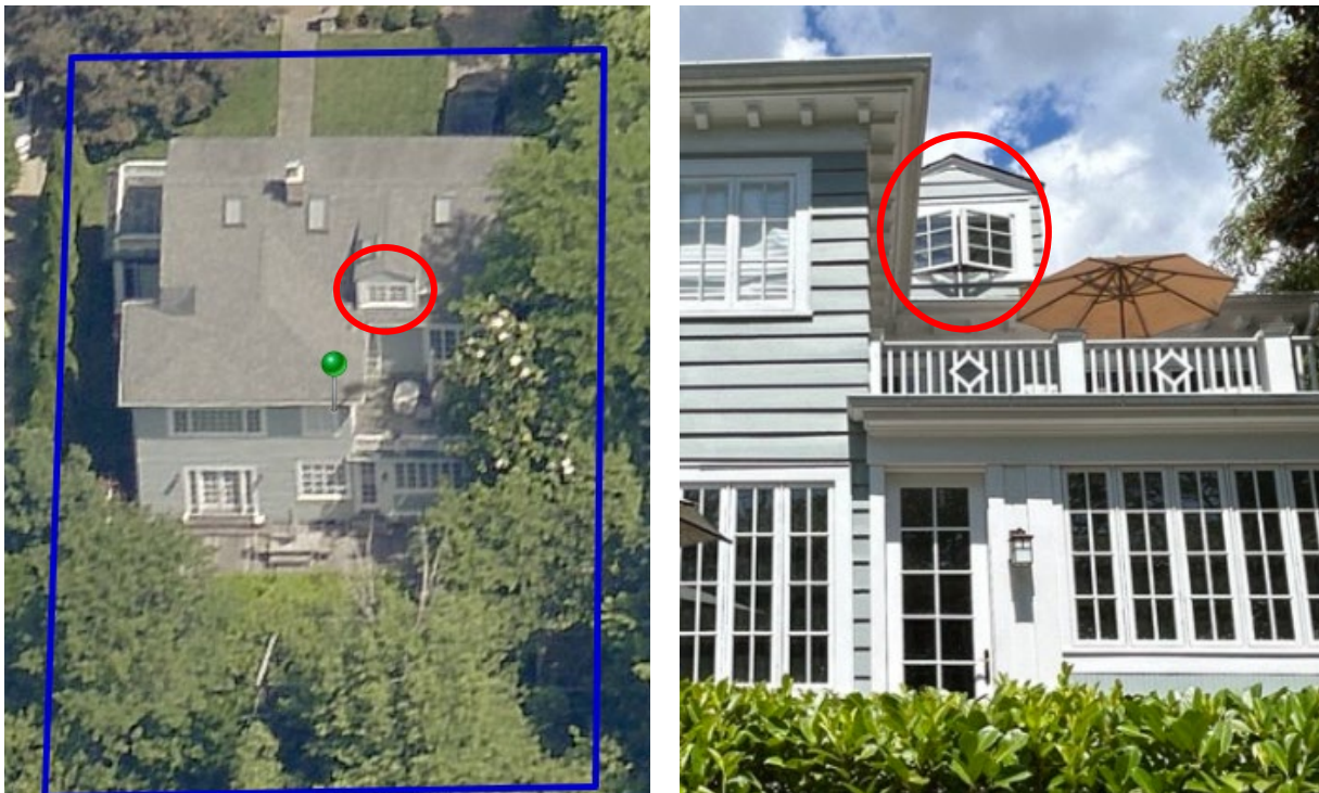
Figure 4: Area of work on the south elevation (left, circled in red), and closer view of the pair of south-facing casement windows to be replaced (right, circled in red).
