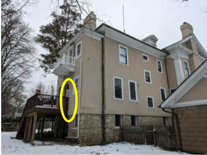
Figure 2: Southeast corner of the house. The arch to be blocked in is circled.
