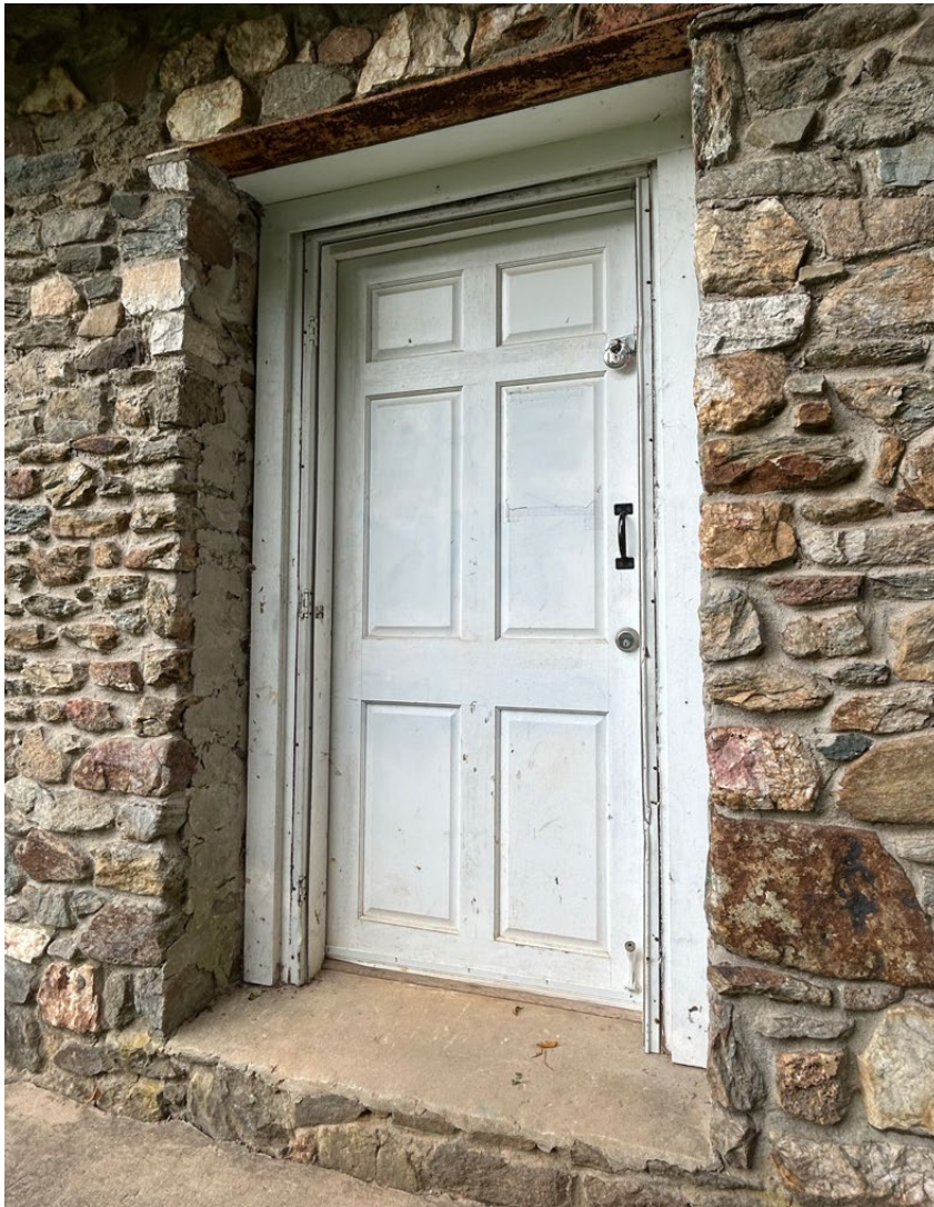
Figure 5: Details of the existing door and framing. Holes, weathering, and scars within the masonry opening suggest that the original door and frame may not have been set as far back in the opening as the existing system.
