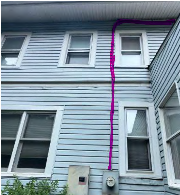
Utility Meter after Install
