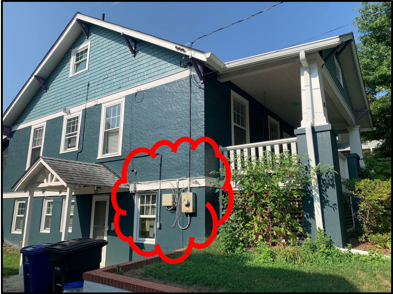
Figure 5: The load center and disconnect switch will be installed on the left-side elevation near the building's existing meter and electrical panel.
