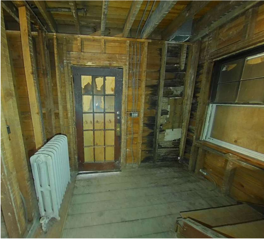
EXISTING DAMAGED FRONT DOOR
