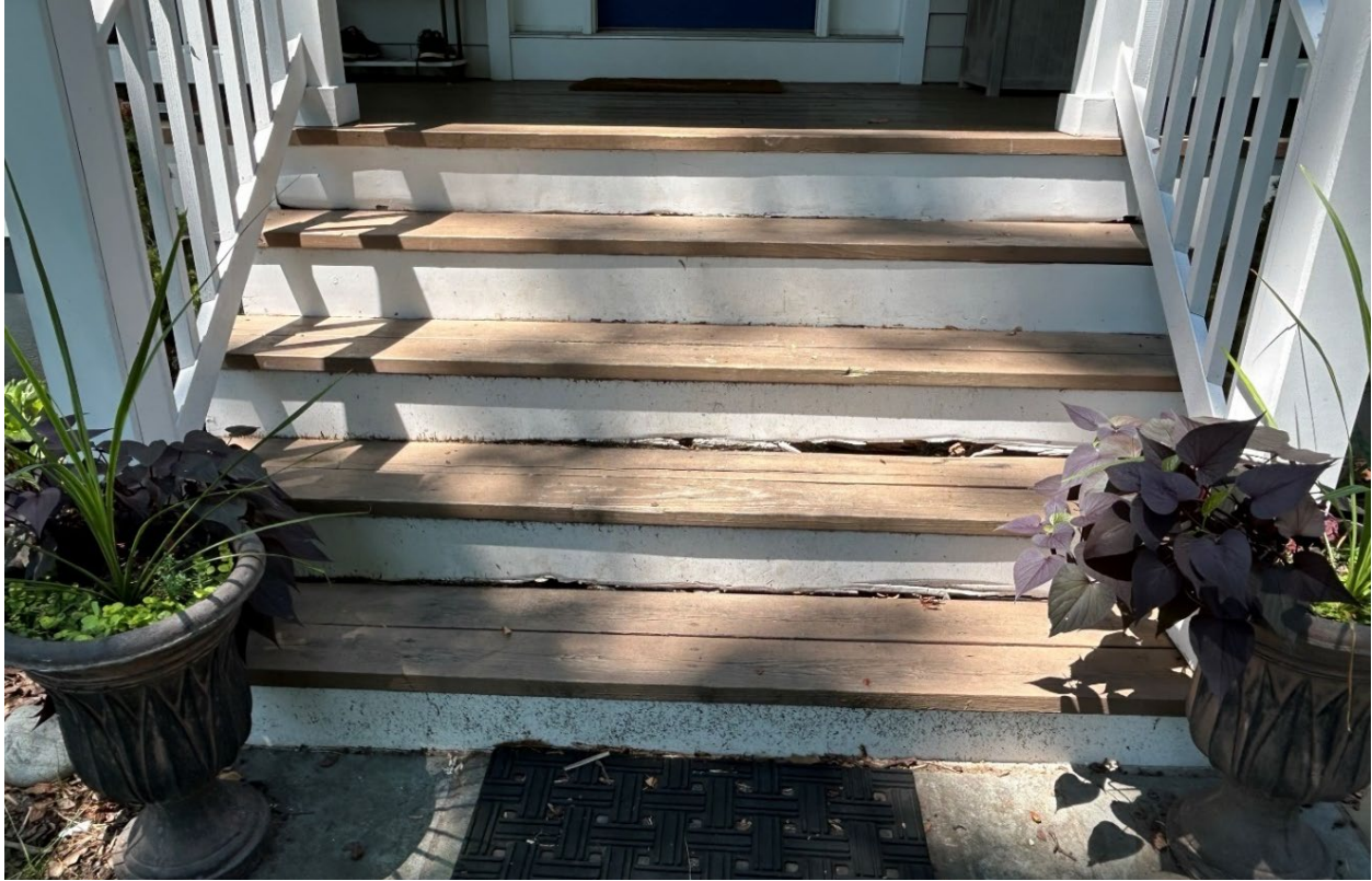
Figure 8: Condition of the front steps, July 2024 (Historic Preservation Office).
