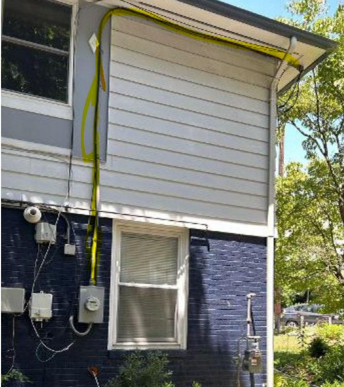
Utility Meter after Install
