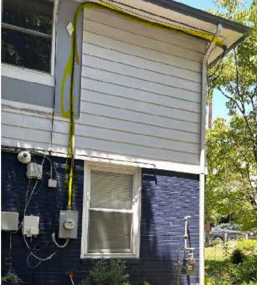
Figure 5: The applicant provided this photo to highlight the location where the load center and disconnect switch will be installed on the east-facing elevation near the building's existing meter and electrical panel.
