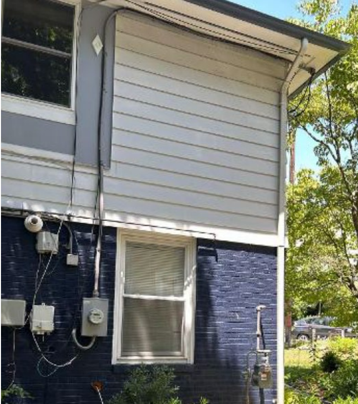
Utility Meter before Install
