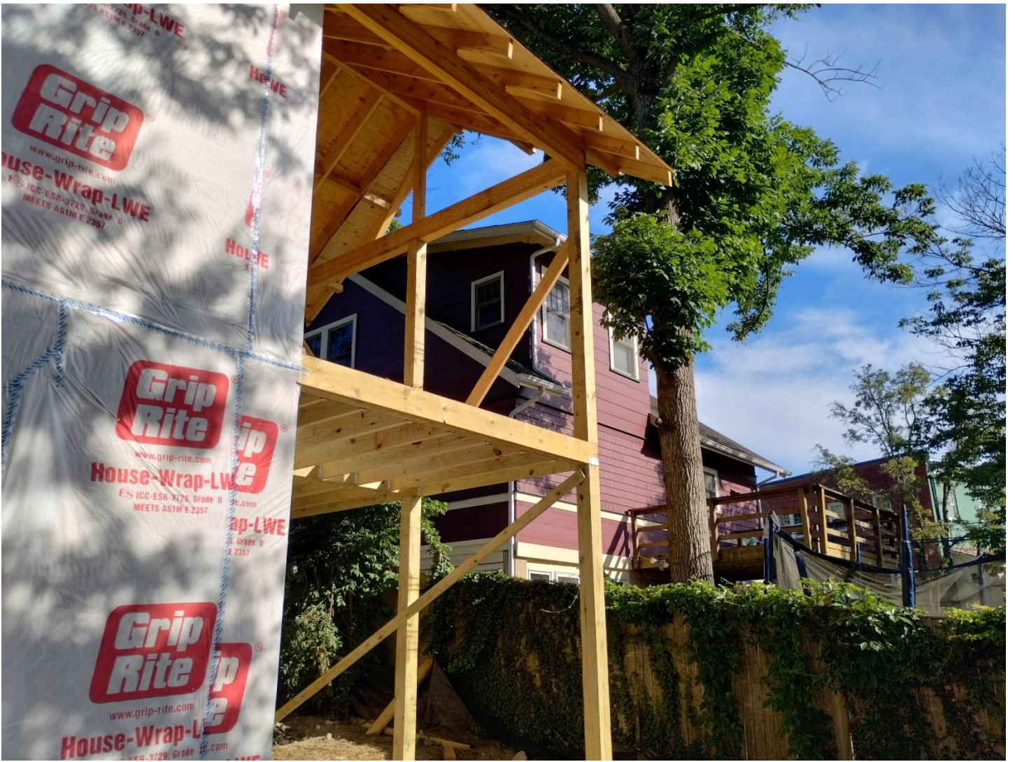
Fence between 7338 Carroll and 7336 Carroll Ave, SW and left side of building. New deck construction in foreground. This length of fence will be replaced with new fence in same style, dimensions and color.
