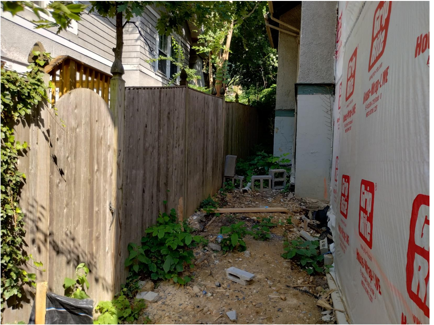
Existing fence on NE (right) side of property, not in scope and will not be changed.
