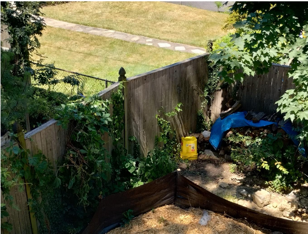
Existing fence on West side corner, will be replaced with new fence in same style, dimensions and color. Note the angles of how fence was originally installed.
