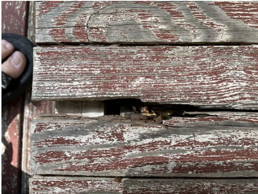
Rotten Porch Flooring
