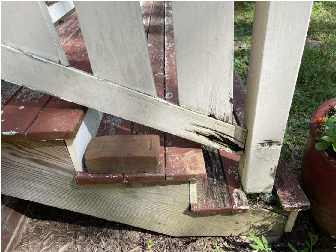
Rotten Porch Railings
