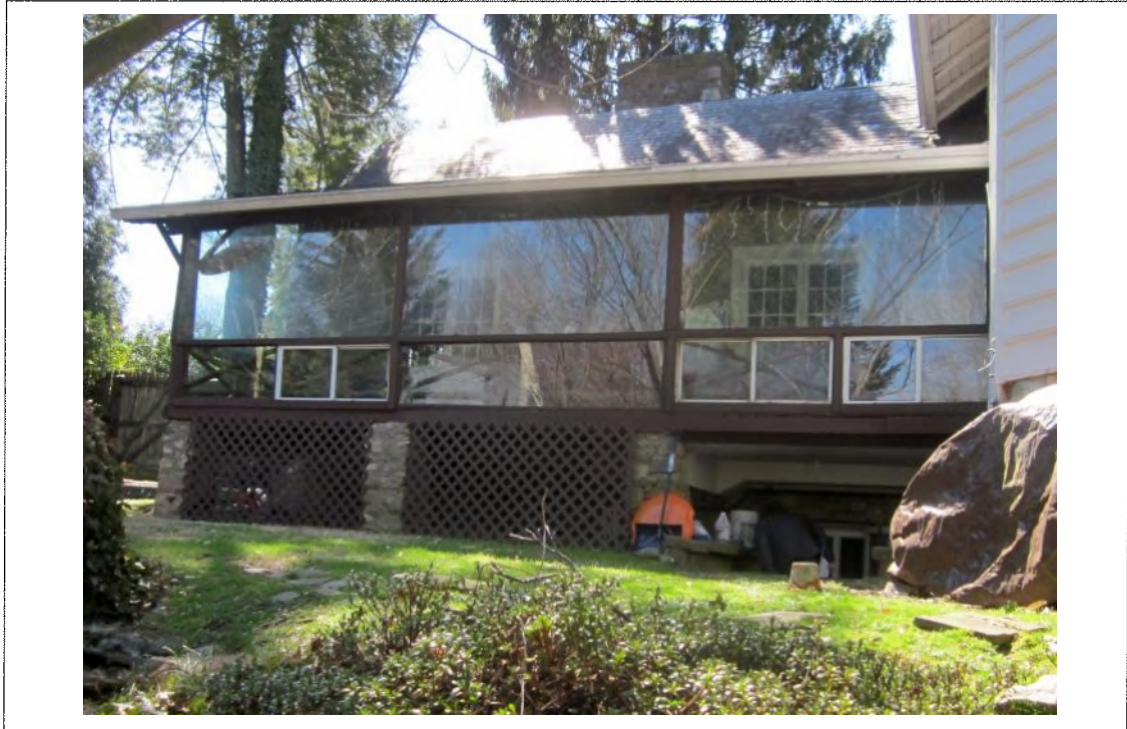
Existing North elevation. Rear porch in poor condition; plexi-glass to be replaced Detail: with insulated glazing and structure to be replaced with new posts to support roof.
