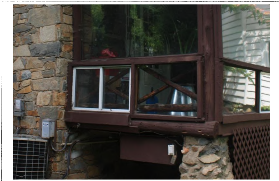
Existing North elevation. Rear porch in poor condition; plexi-glass to be replaced Detail: with insulated glazing and structure to be replaced with new posts to support roof.
