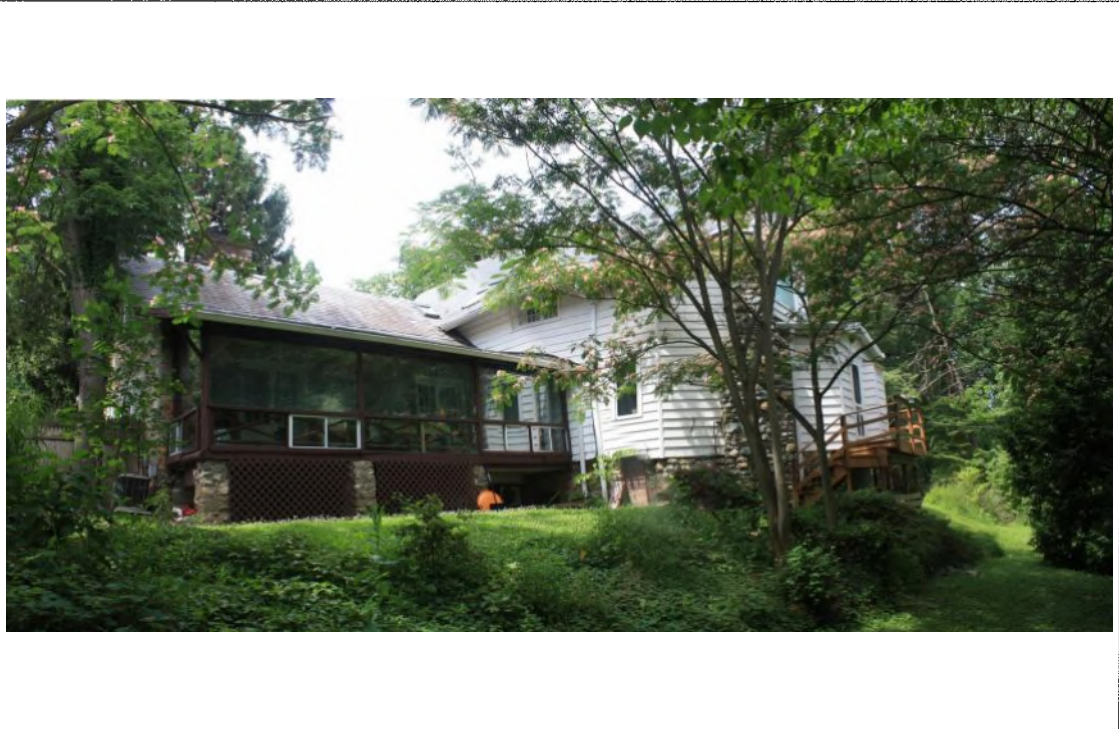
Existing North elevation. Rear porch in poor condition; plexi-glass to be replaced Detail: with insulated glazing and structure to be replaced with new posts to support roof.
