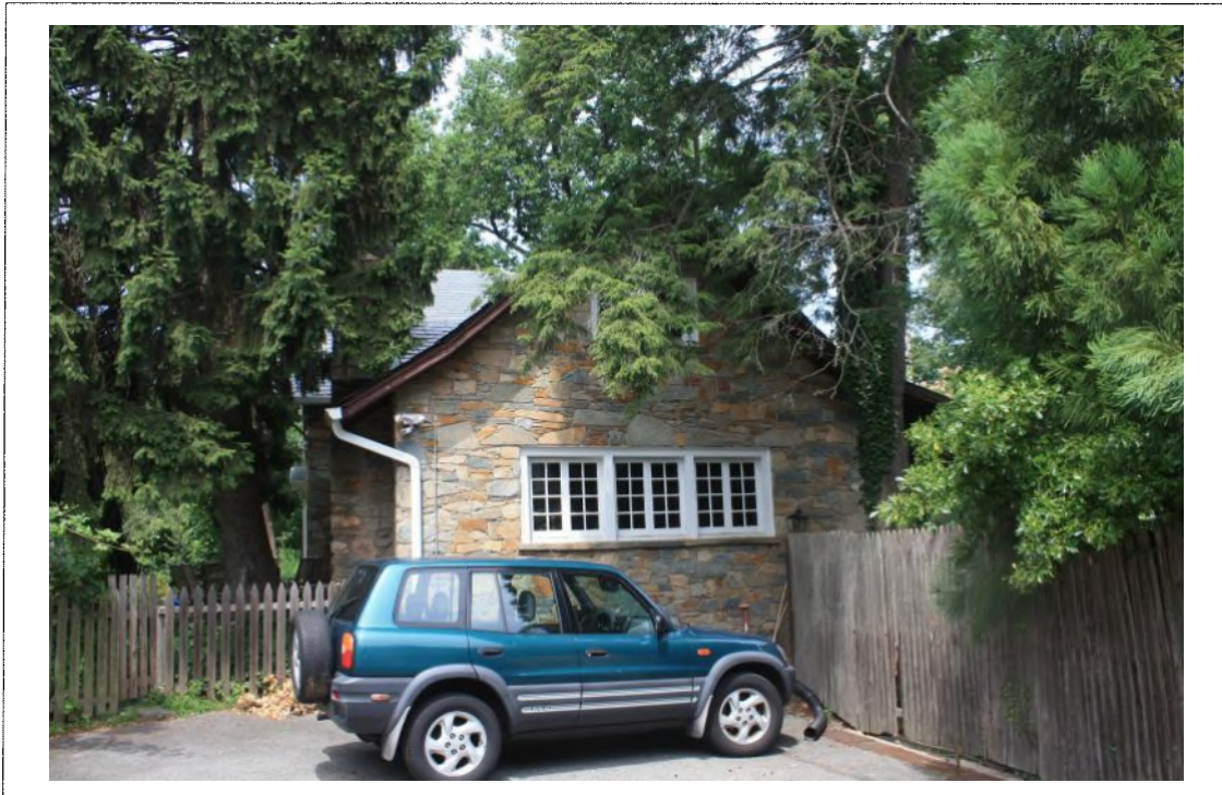
Existing East elevation. Terrace to be extended to south (not pictured); Detail: rear porch glazing to be replaced (see previous image).
