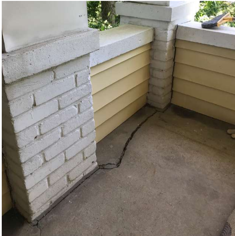
Detail: 7017 SYCAMORE AVE. CRACKED PORCH SLAB
