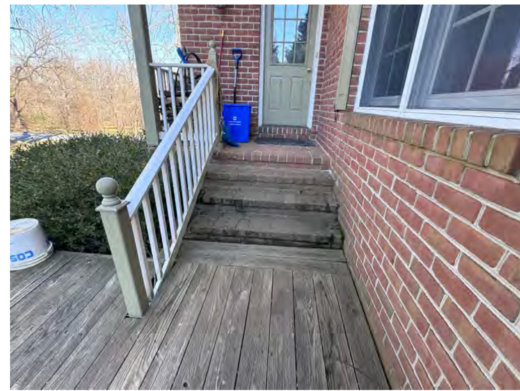
Existing Brick Steps @ Deck to Remain. Shorten Ex. Handrail and move Bottom Post
