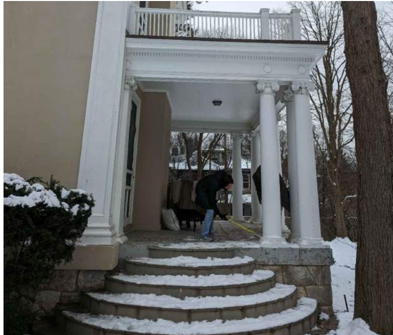
EXG. NON-HISTORIC FRONT STEPS TO RIGHT SIDE PORTICO
