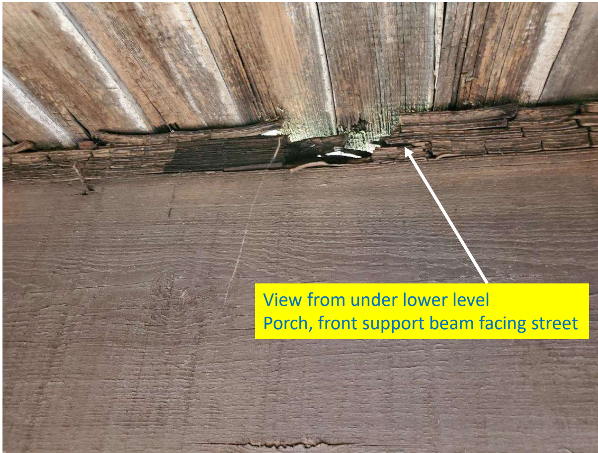
Photo 11 - 7102 Maple Ave – lower porch floor joist rot
