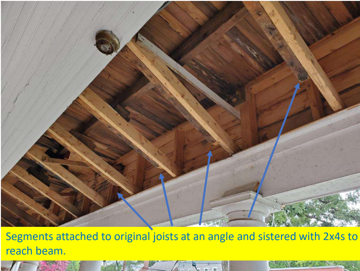
Photo 1 - 7102 Maple Ave – cut joists too short
