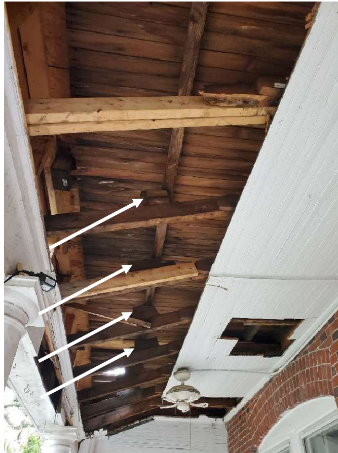
Photo 15 - 7102 Maple Ave – odd shaped shims holding up 20 Foot long 2x4s
