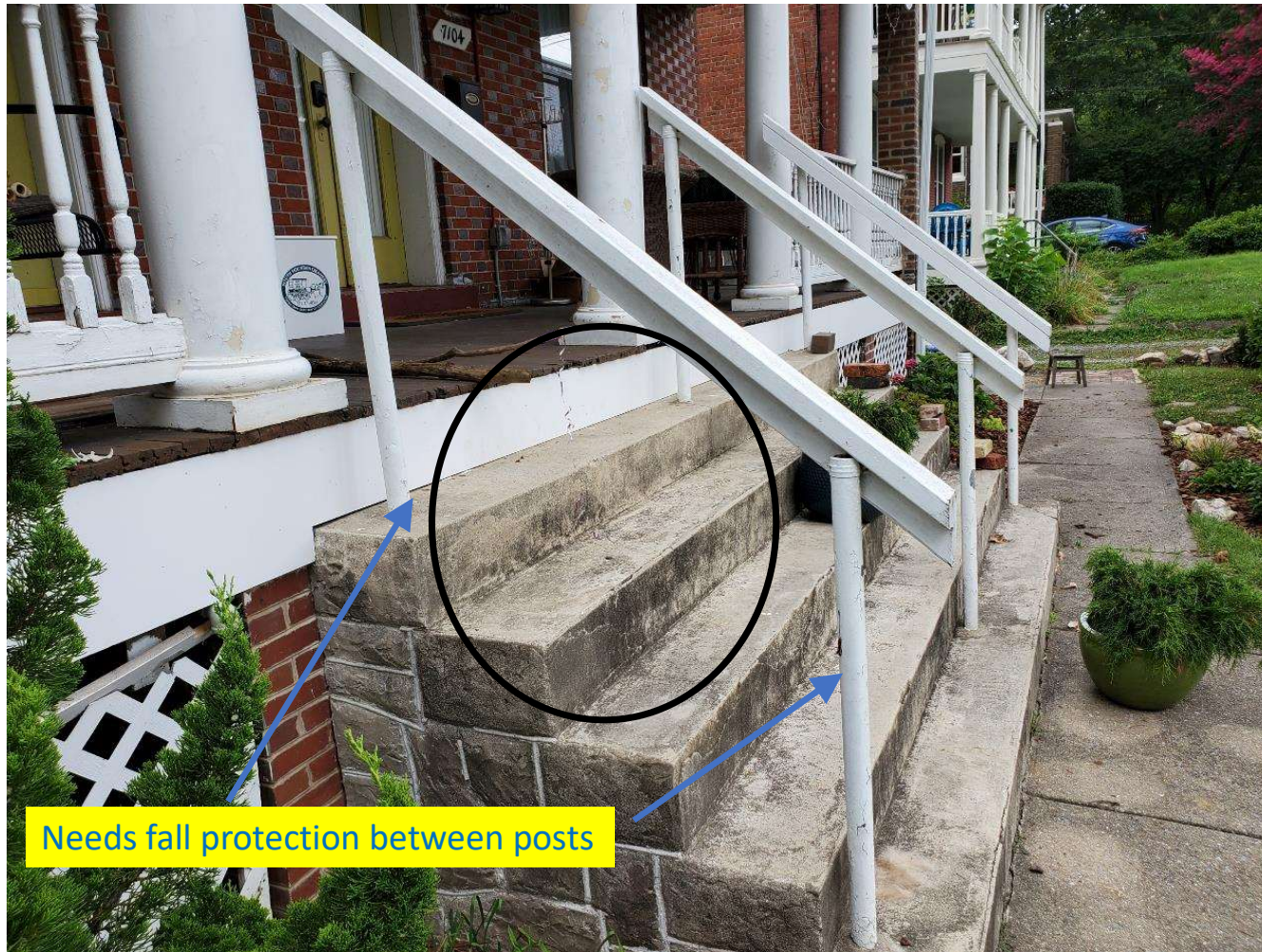
Photo 14 - 7102 Maple Ave – steps showing no fall protection
