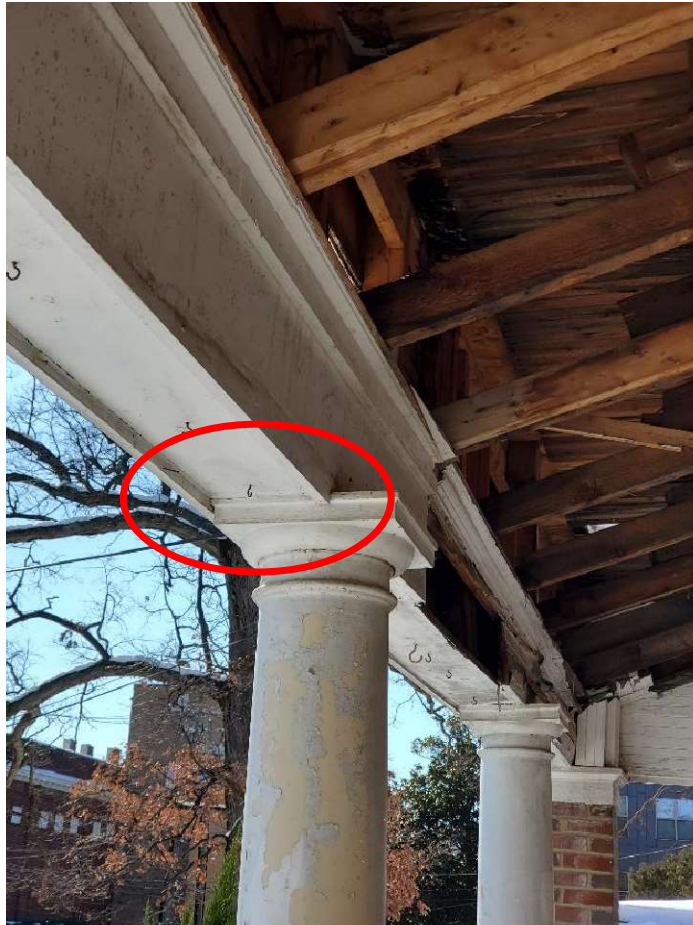
Photo 10 - 7102 Maple Ave – off center beam
