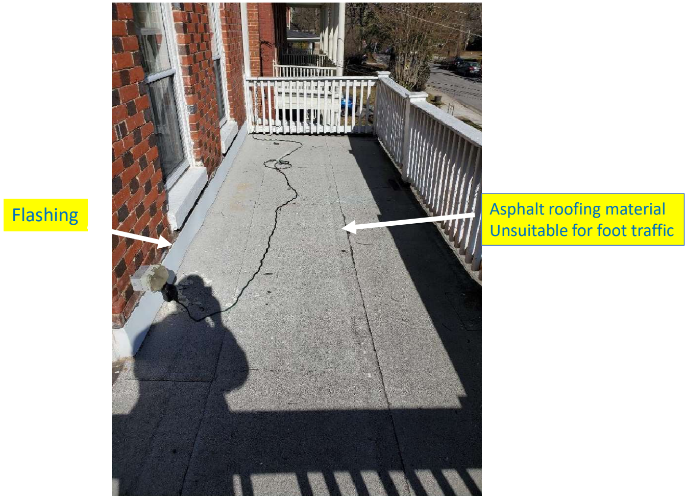
Photo 7 - 7102 Maple Ave – Asphalt roofing material
