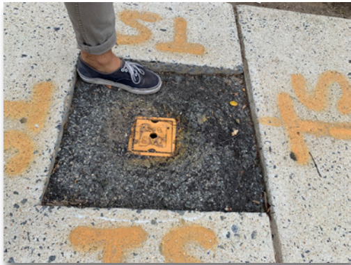
A poorly filled utility cut in the sidewalk. Shoe for scale.
