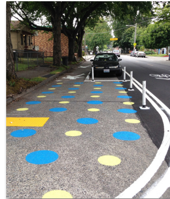
A painted pedestrian pathway in the street is separated from traffic by parked cars, temporary concrete curbs, and white flex posts. Photo Credit: Dongho Chang
