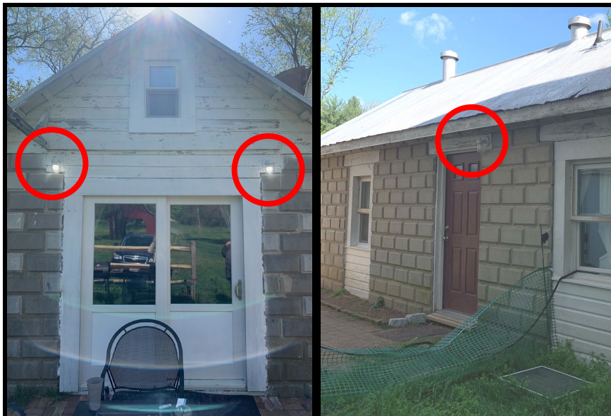
Figure 15: The sliding composite doors on the front elevation, left, and the fiberglass door on the right-side elevation. The lights are circled in red.
