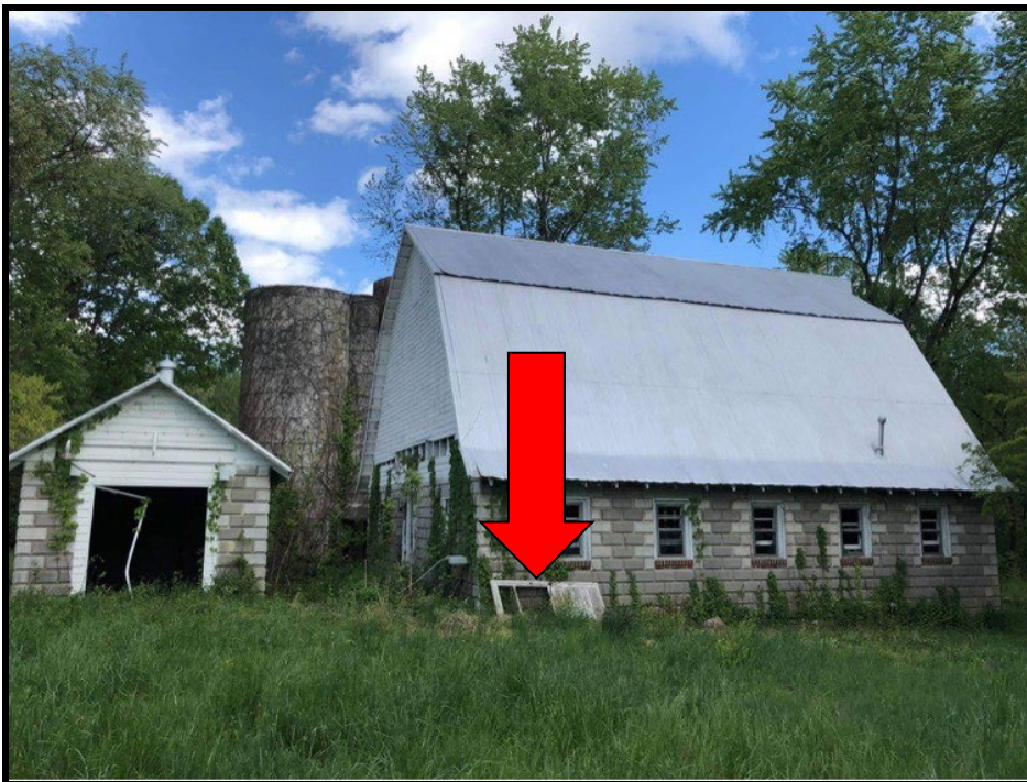
Figure 13: The applicant provided this circa 2021 photo of the Milk House and Dairy Barn. The arrow points to what appears to be a wood screened door that may have been installed on the Milk House or Dairy Barn.
