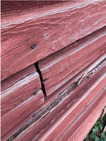
Detail of deteriorated siding.
