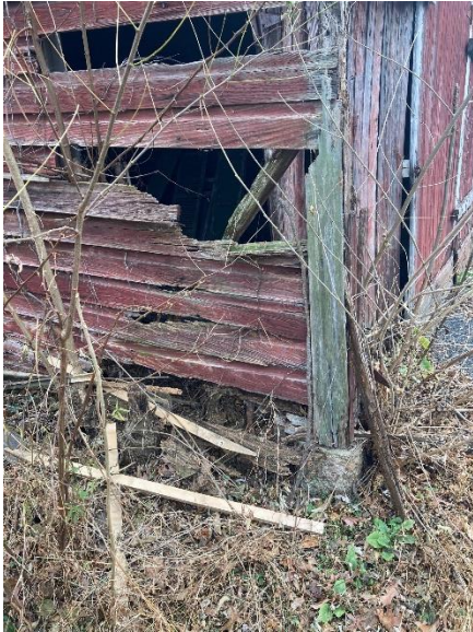
Detail of substandard, footer, rotted on-ground sill plate, and siding and corner post.
