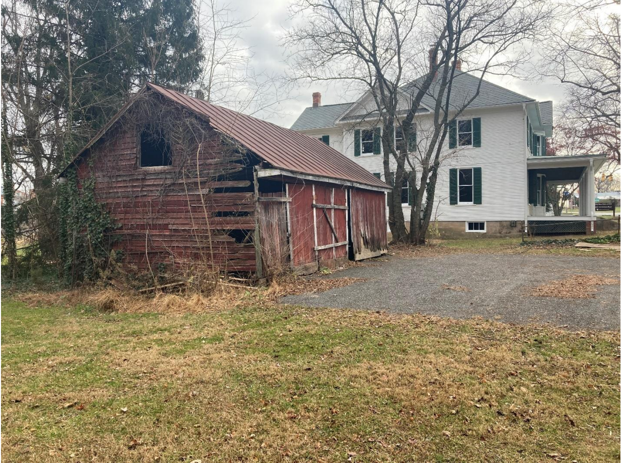
North elevation, showing deteriorated siding and barn doors and missing window in gable end.
