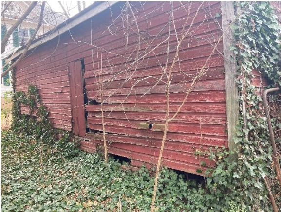
East (rear) elevation with north bay in foreground; south bay at rear.
