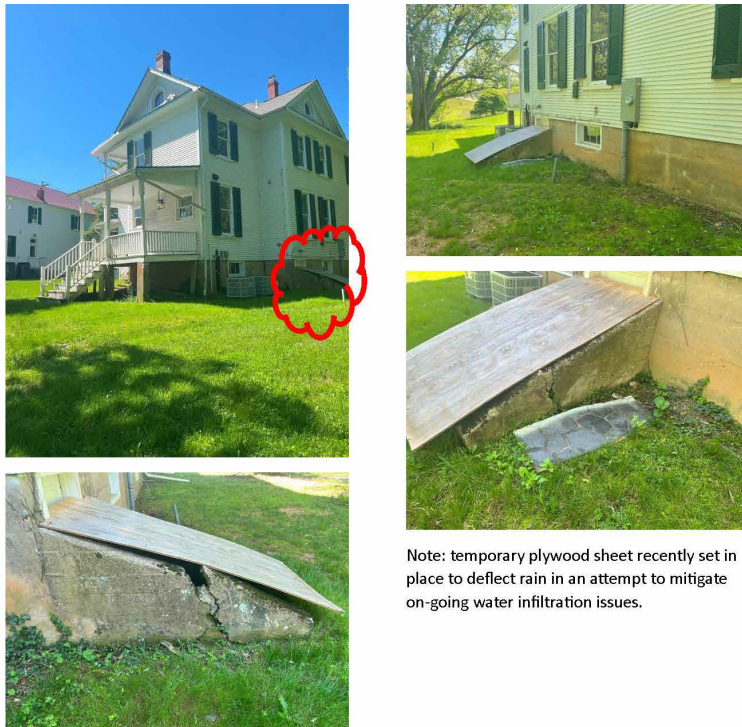
Figure 7: The applicant provided these photos showing the areaway on the left-side elevation.
