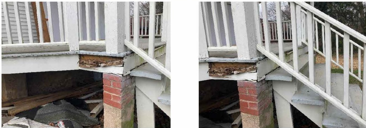
Figure 2: The applicant provided these photos showing the condition of the rear porches.
