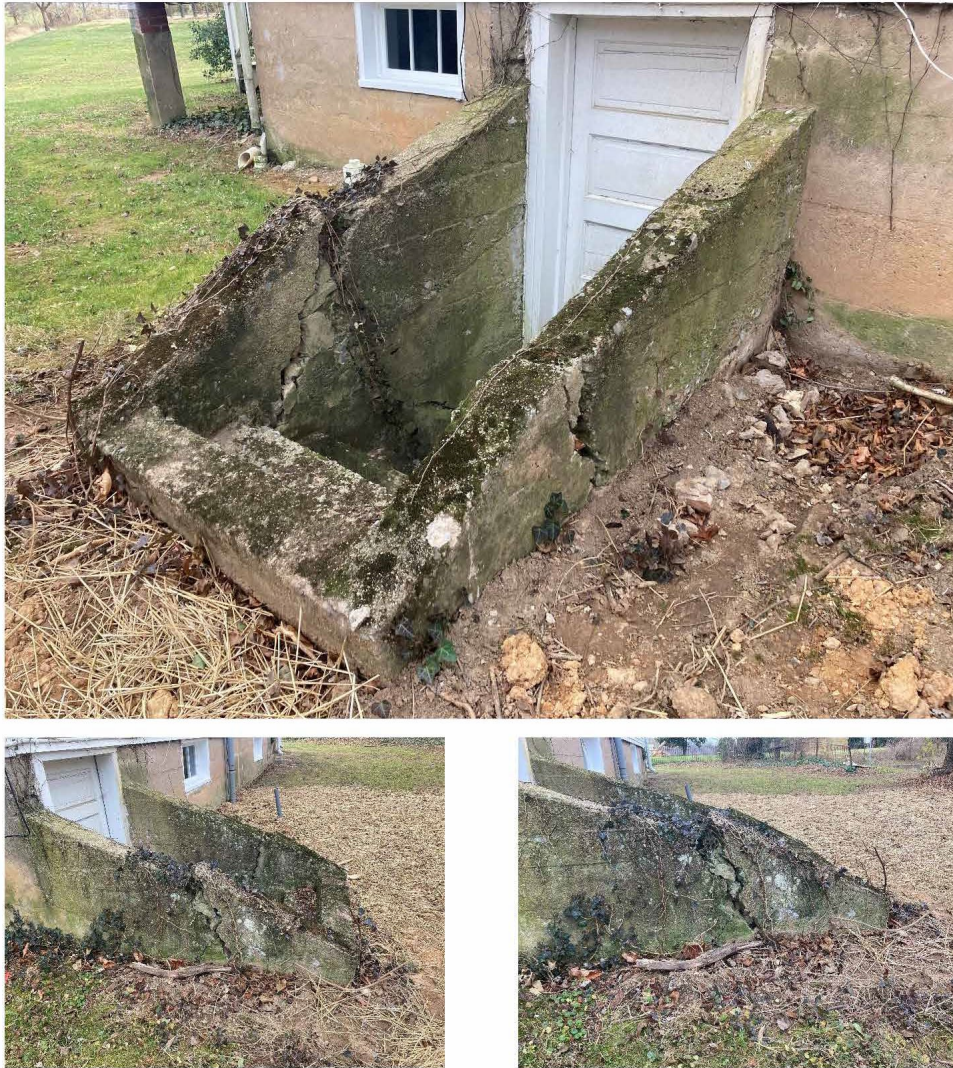
Figure 8: The applicant provided these photos showing the areaway on the left-side elevation.
