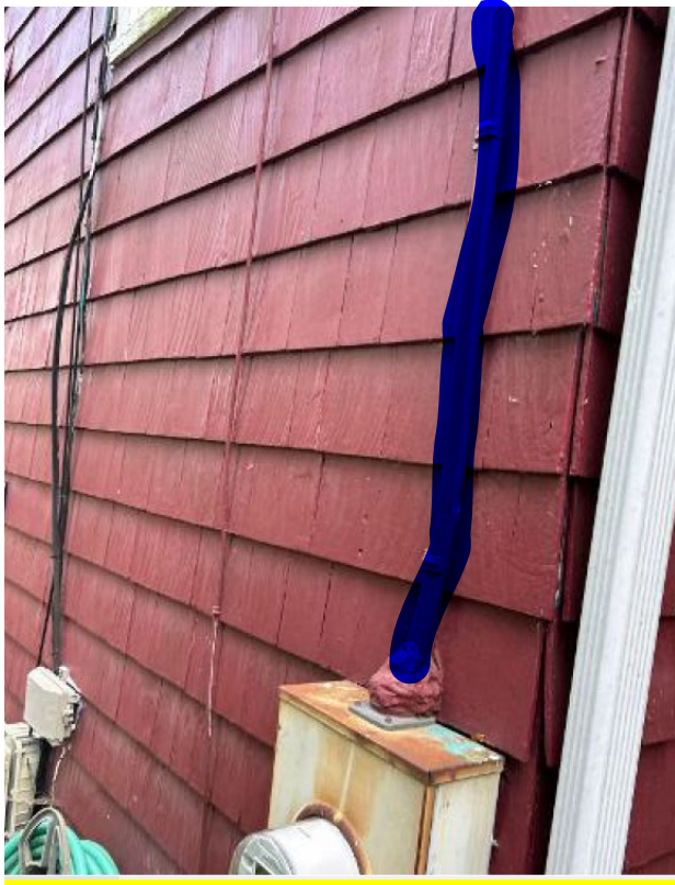
Utility Meter After
