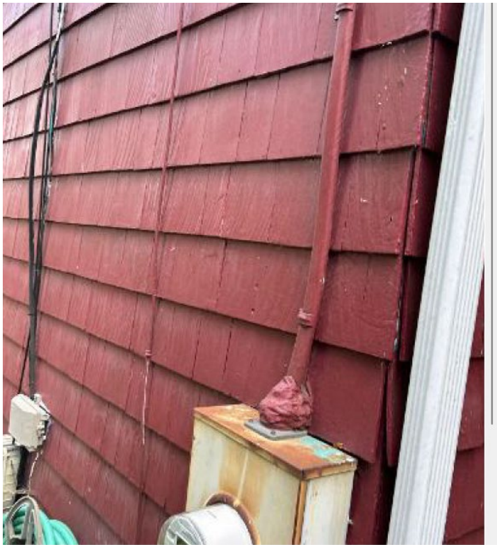
Utility Meter Before
