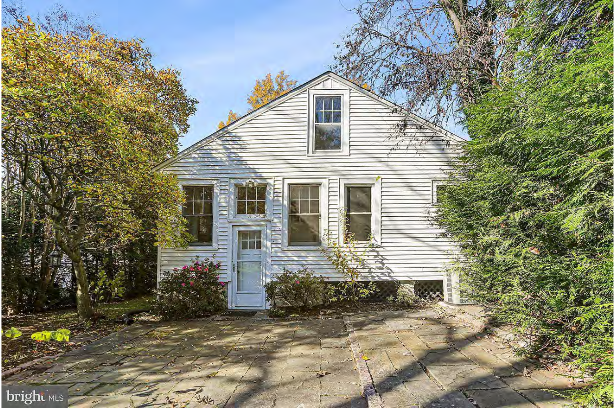
REAR FACADE SHOT . NOTICE BUILDING ON RIGHT IS ON PIERS. WHEN PROPOSED ADDITION PLACED DRAINAGE/GRADE OF CREATED OPEN CRAWLSPACE TO BE VERIFIED AND ADDRESSED. SHOULD REMAIN AS EXISTING CONDITION UNLESS SOME REGRADING REQUIRED
