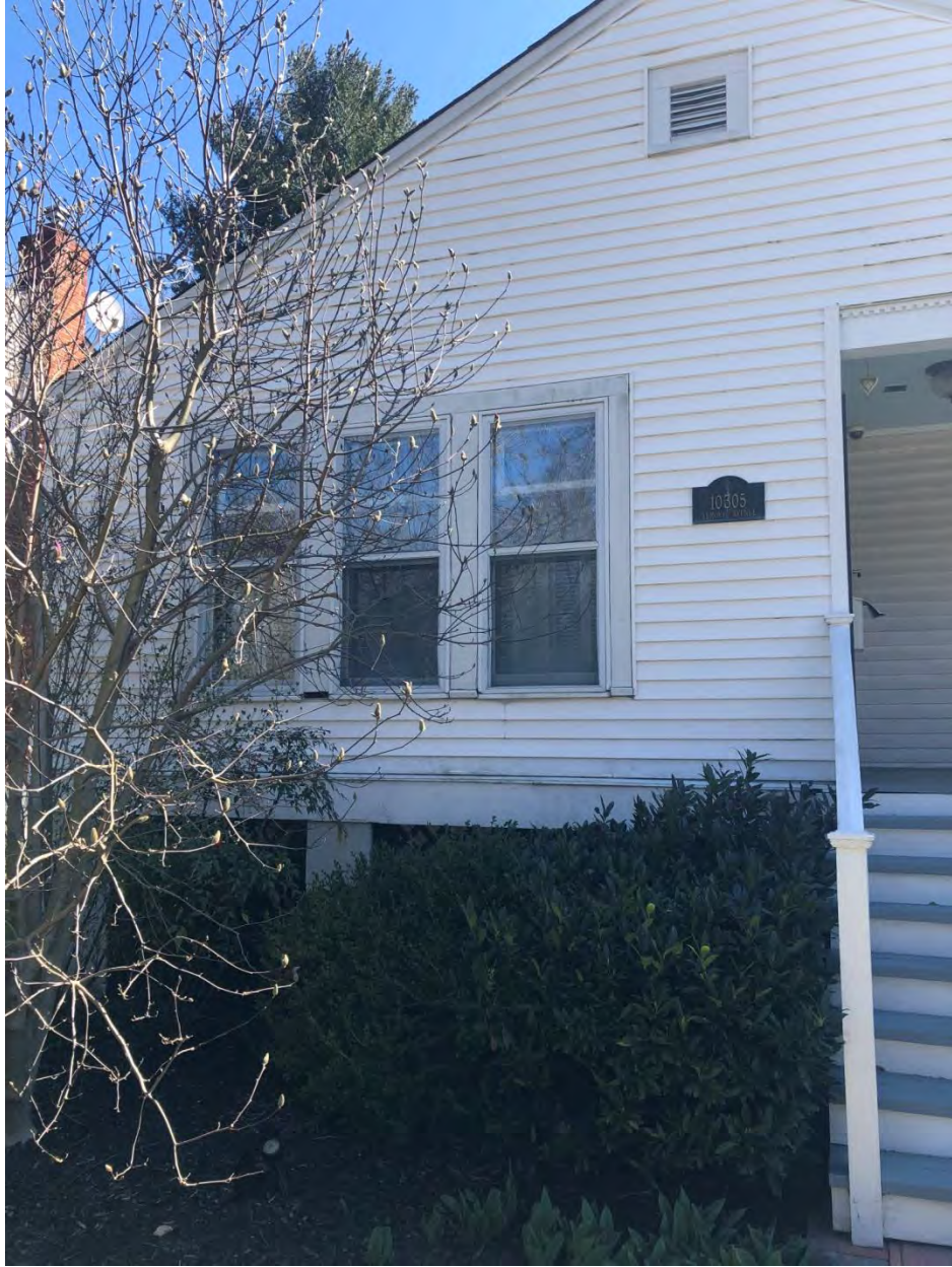
CURRENT LIVING RM WINDOW PHOTO. LATTICE TO BE REPLACED.
