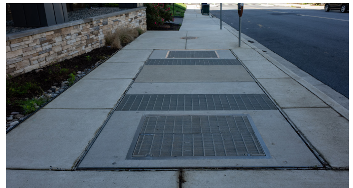
Figure 3-13. Example of grates that may present tripping hazards
