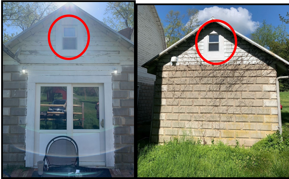
Figure 11: The openings and windows newly installed in the gable ends are circled.
