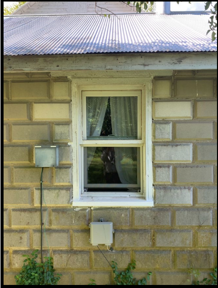
Figure 14: A representative photo of the one of the newly installed windows with the previous upper wood sash intact.
