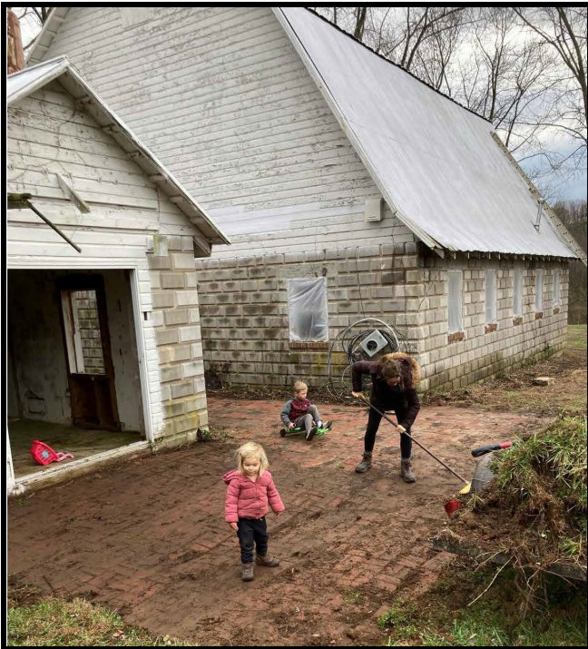
Figure 9: The applicant provided this photo taken after he took ownership in October 2021 to show the Milk House with no front door and window removed on the right-side elevation.
