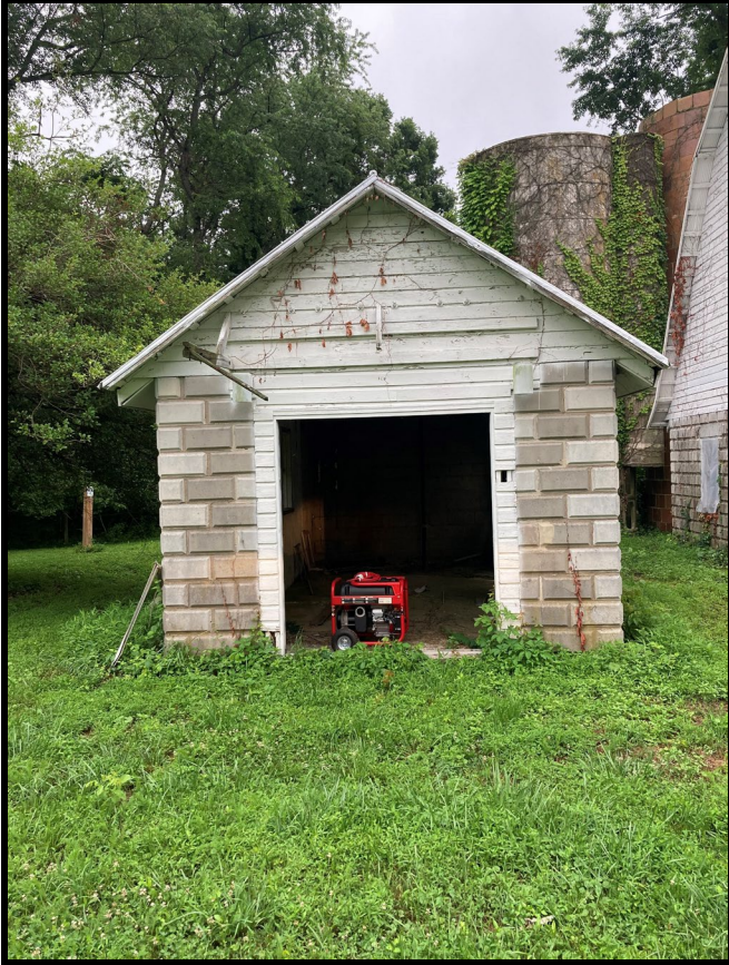
Figure 8: The applicant provided this photo taken after he took ownership in October 2021 to show the Milk House with the previous front doors removed.
