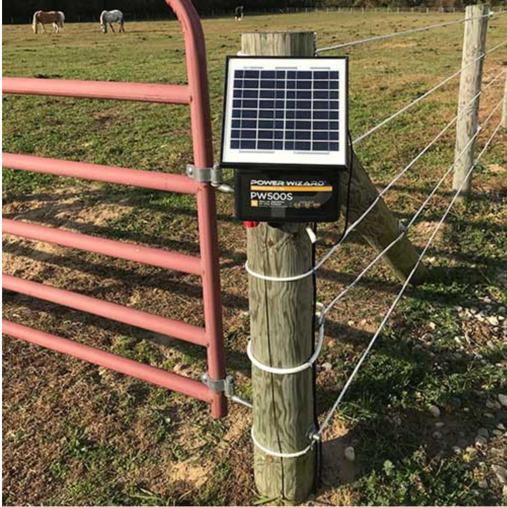
Typical solar charger used for electrifying agricultural fences.
