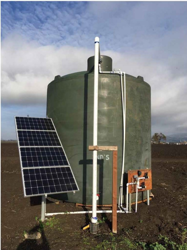
Figure 5: The plastic water storage tank will measure 7-feet wide and 9-feet tall and be solar powered.
