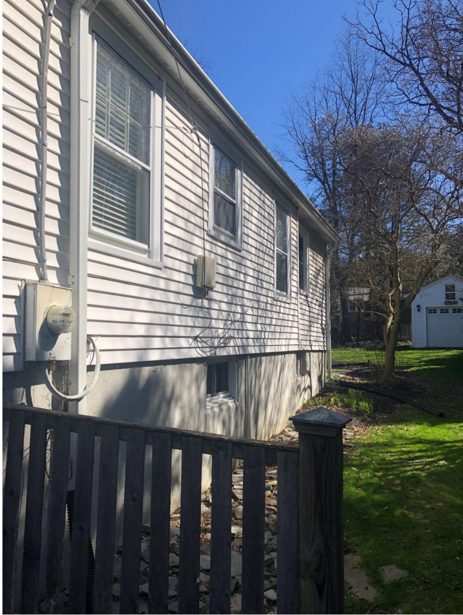
SOUTH FACADE WITH VIEW OF TREE TO BE REMOVED. SEE DRAINAGE NOTE BELOW
