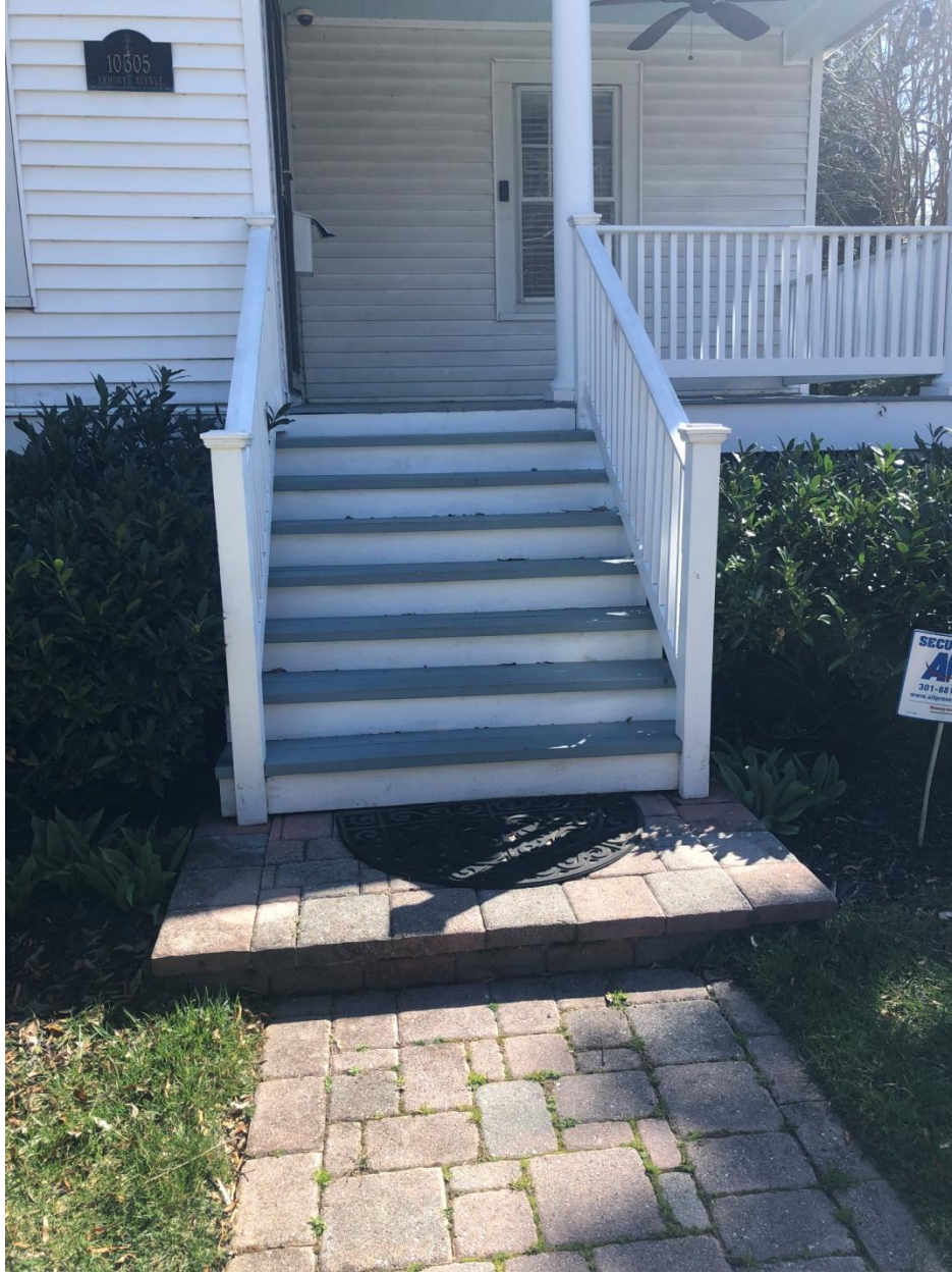
CLOSE UP SHOT OF FRONT STAIRS...RAILING REMAINS , PAVERS REMAIN. STAIR TREADS PROPOSED WITH NEW TREX REPLACEMENT (MAY REQUIRE RESTRUCTURING STAIR UNDERNEATH)
