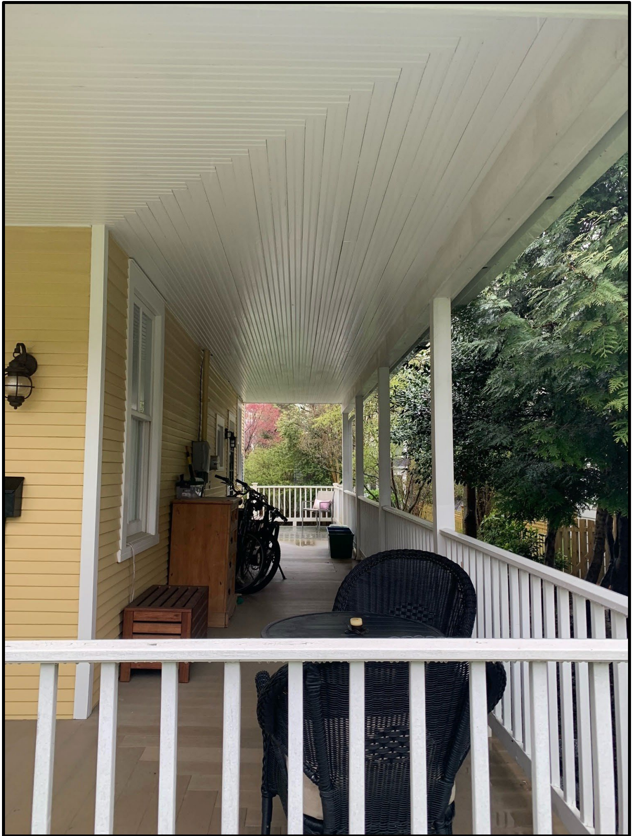
Figure 4: The existing wraparound porch at 3705 Underwood St. The 9-foot long section toward the far end is proposed to be enclosed.
