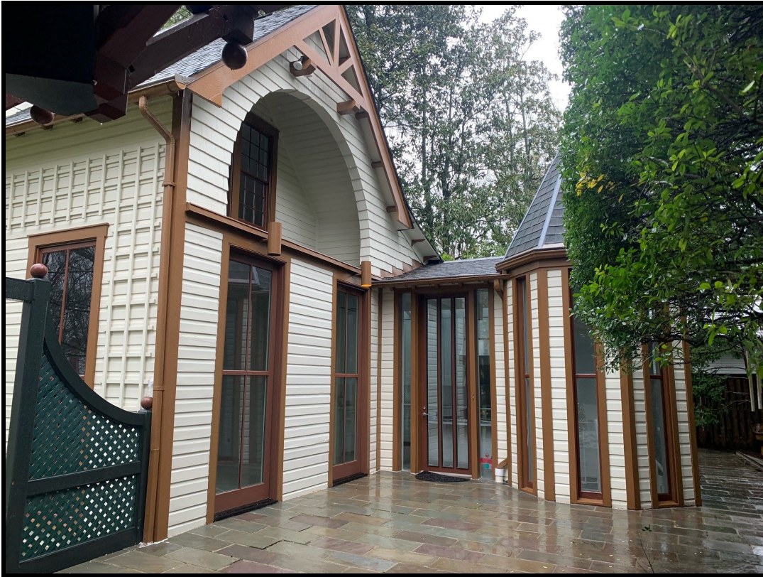
Figure 5: The octagonal room and hyphen on the right-side elevation will be demolished to accommodate the two-story addition.
