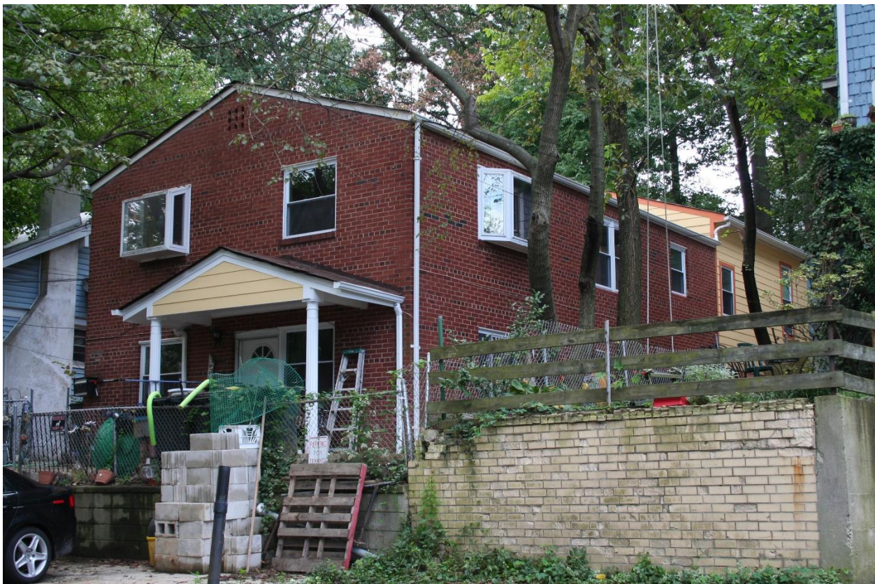
Figure 5: Photo showing the failing brick retaining wall (right) and the house at 6708 Westmoreland (left).
