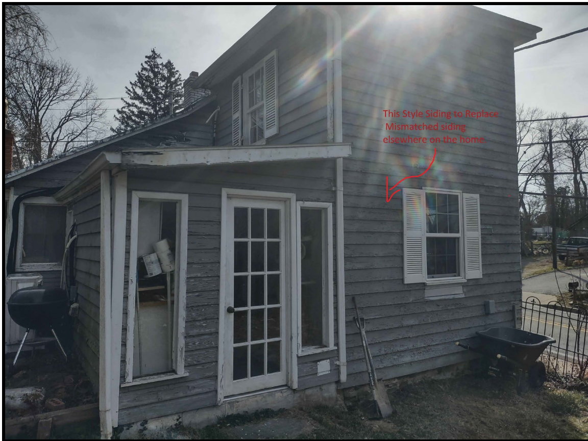
Figure 5: The applicant provided this annotated photo of the left-side elevation to show the siding to be installed on the entire building.
