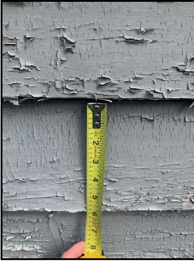
Figure 6: The siding proposed for the entire building will have a 6-inch reveal to match the siding on the left-side elevation.
