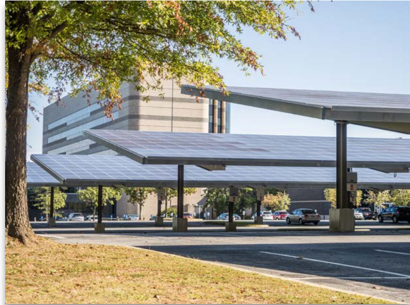
Parking lot at Verizon offices with shade and solar panels
