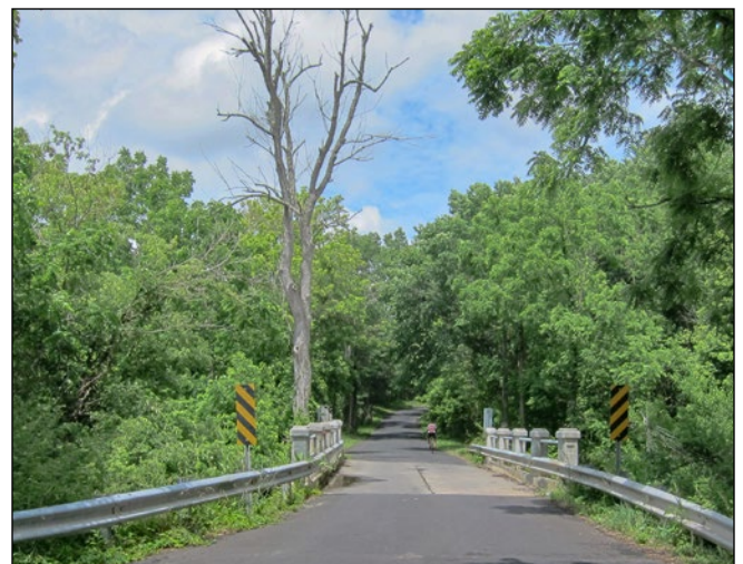
Looking east on Schaeffer Road toward the 1925 one-lane pipe bridge over Little Seneca Creek
