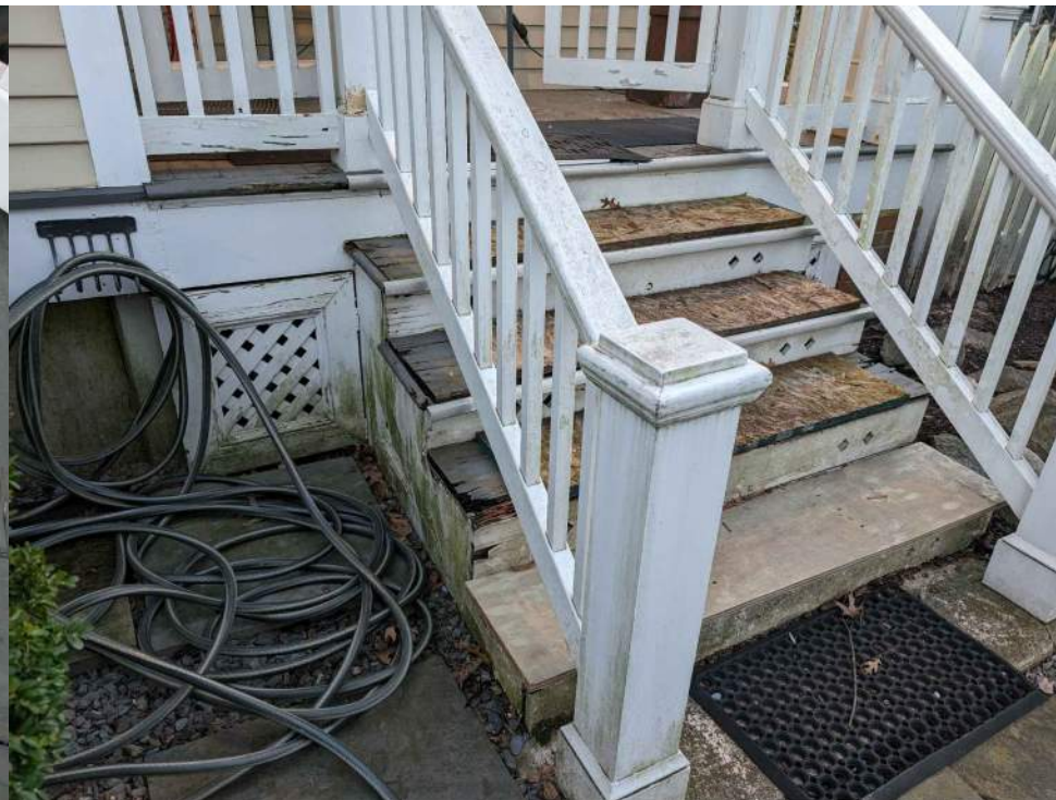
DETERIORATING SIDE PORCH STEPS AND RAILINGS
