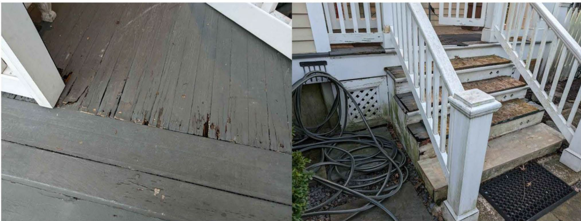
ROTTING DECK BOARDS AT FRONT PORCH
