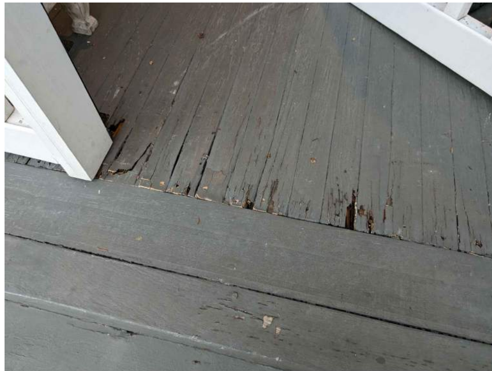
ROTTING DECK BOARDS AT FRONT PORCH
