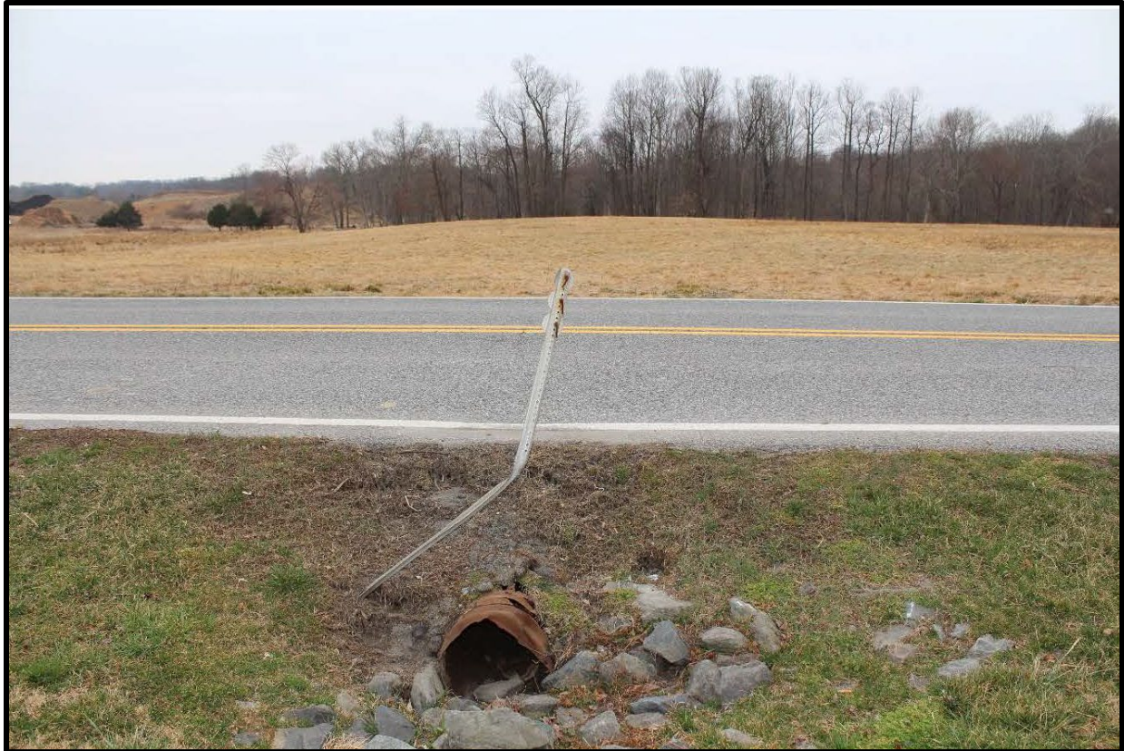
Figure 4: This culvert near the Woodlawn Master Plan Historic Site will be replaced with a stormdrain.
