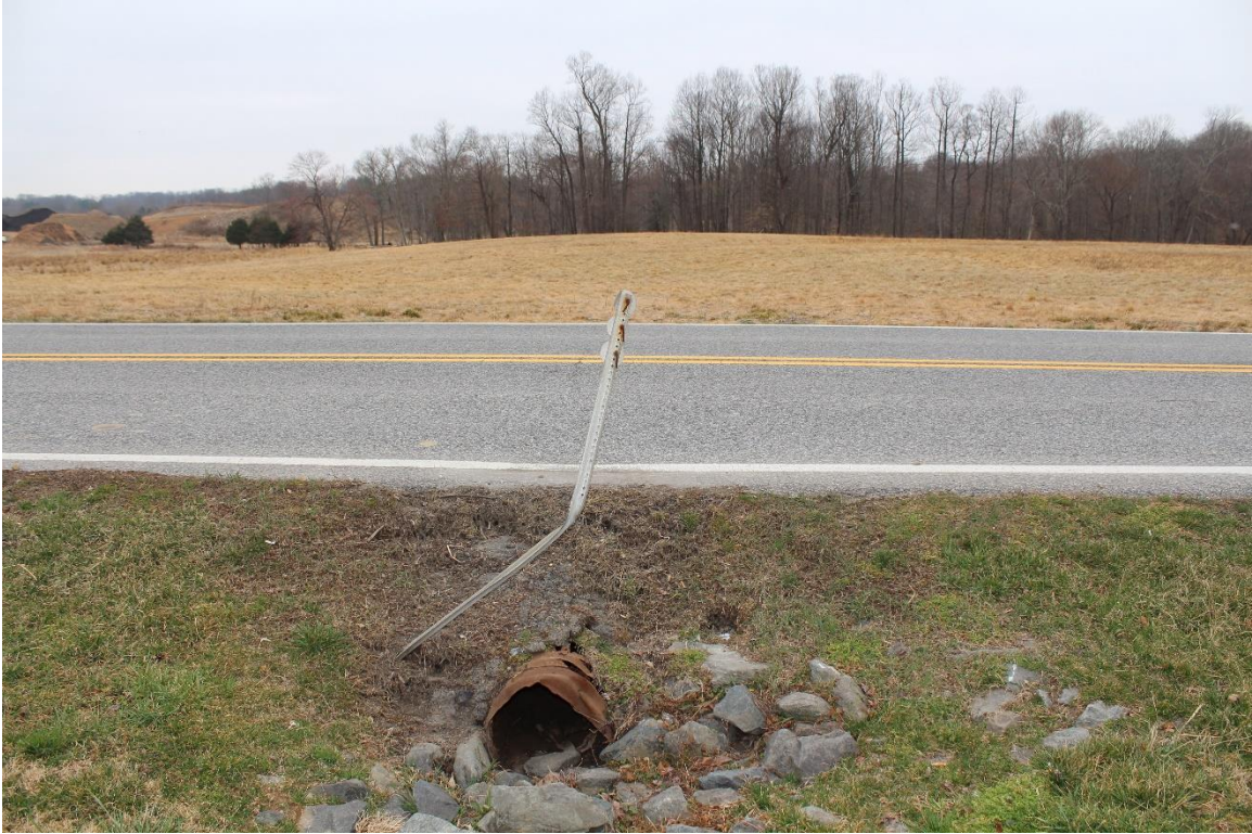
Photo 7: Existing culvert south of driveway, looking southwest to the Red Door Store Property (RK&K, March 2021)
