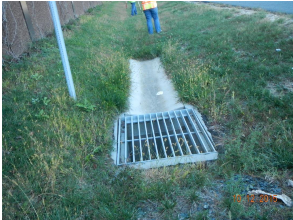
Photo 1: Example of a K inlet with concrete gutter. Note that the gutter is not used for all K inlets and where it is used, it may be used on both sides.
