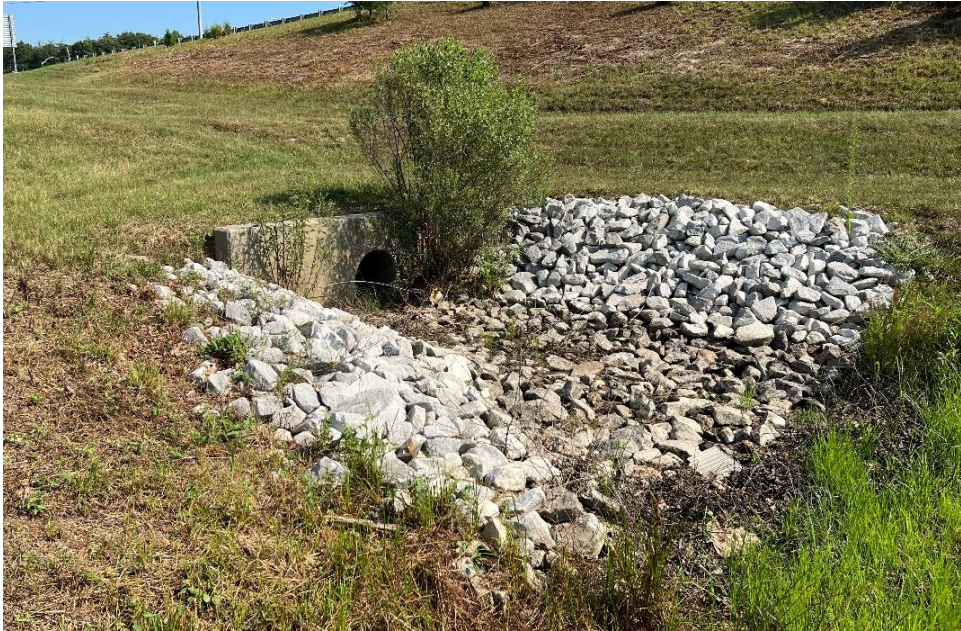
Photo 4: Example of type C endwall with outfall protection.
