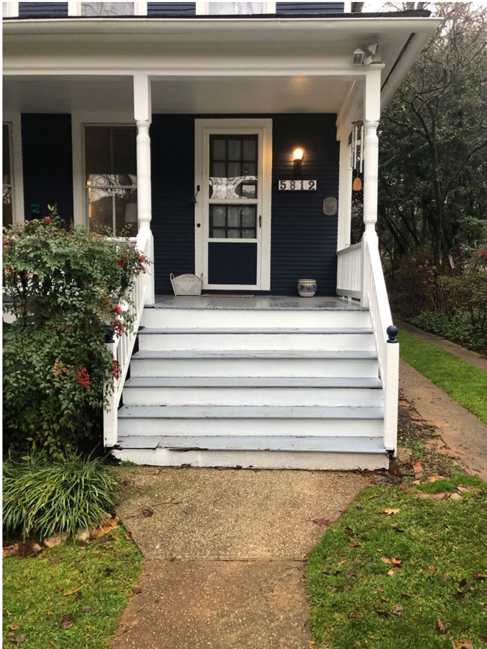
Zoomed in picture of stairs. Deteriorated bottom step visible. Rotted and missing wood seen on bottom step.
