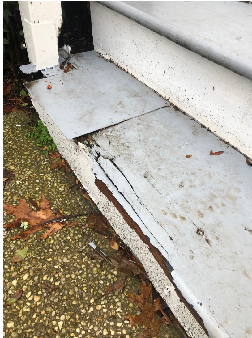
Rotted bottom step. 1 ft by 1 ft metal cover – installed by former owner – visible.
