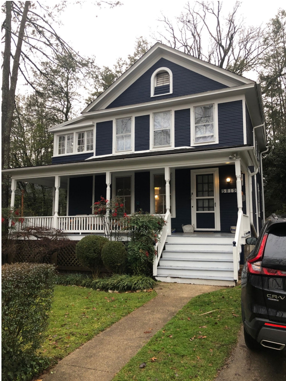
Front view of 5812 Warwick. Deteriorated stairs seen connecting walkway to front door.
