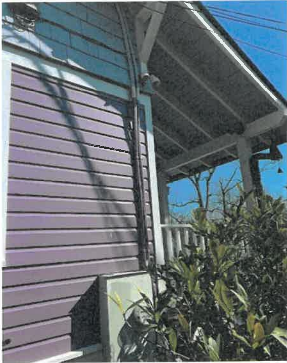
Utility Meter Before Installation
