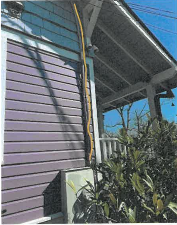
Utility Meter After Installation
