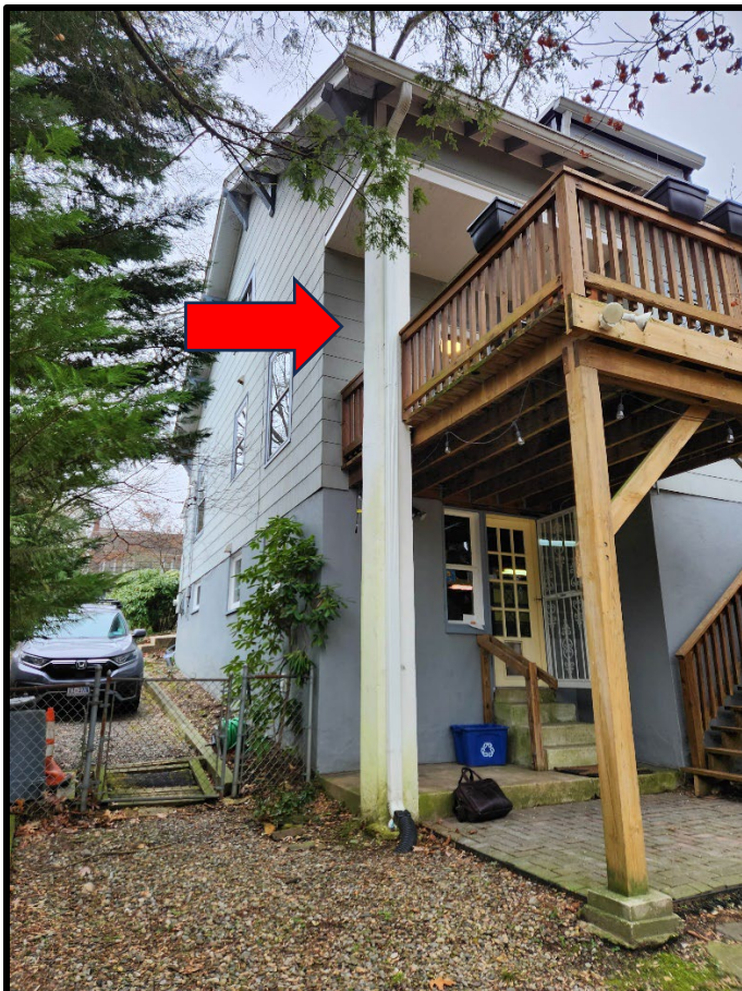
Figure 5: The kitchen will be extended to fill the area between the wall edge and the rectangular post.
