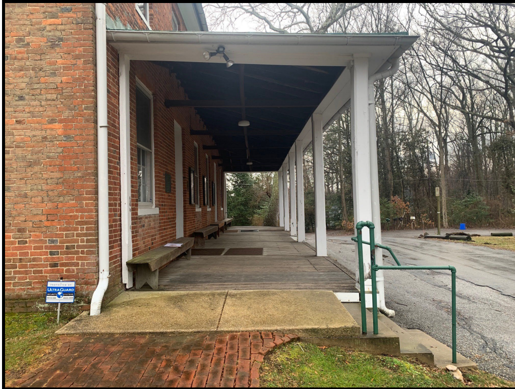
Figure 11: The concrete pad will be replaced with brick pavers and a new concrete stair with railing will be installed.
