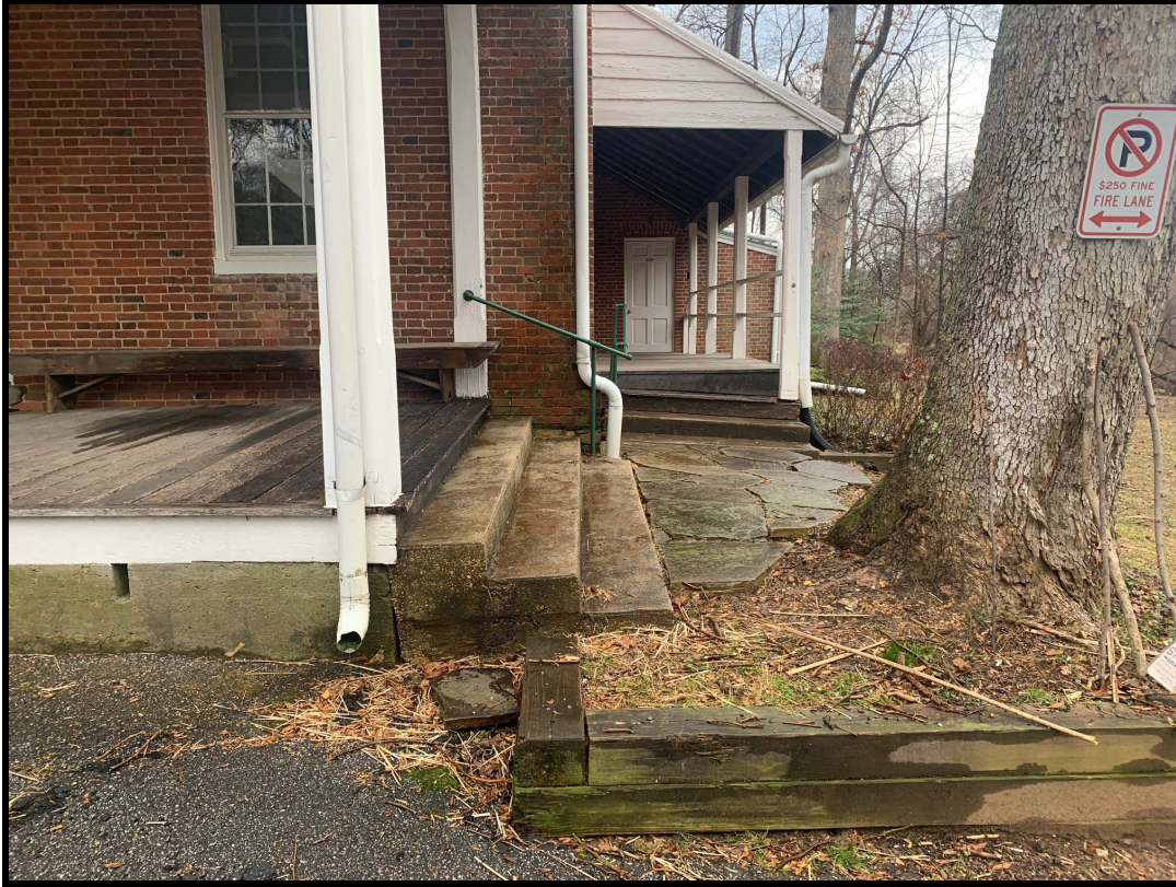
Figure 6. The deck will be installed at this location to link the front porch, left, and the south porch. The tree will remain.
