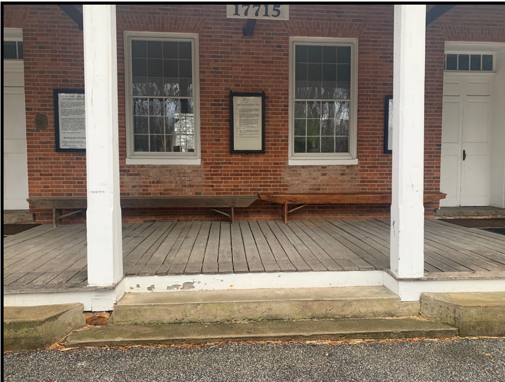
Figure 3. The central concrete stair proposed for replacement is evident in this photo. The concrete steps also proposed for replacement are visible to either side.
