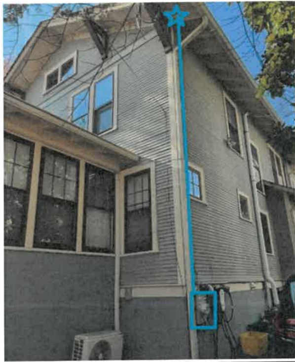
Utility Meter after Installation
