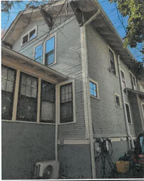
Utility Meter before Installation
