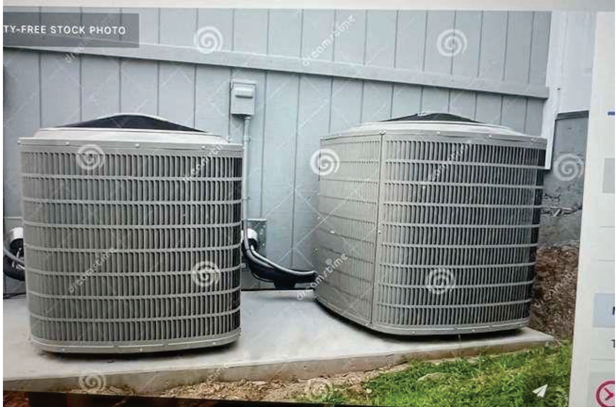
Sample photo of the AC units
