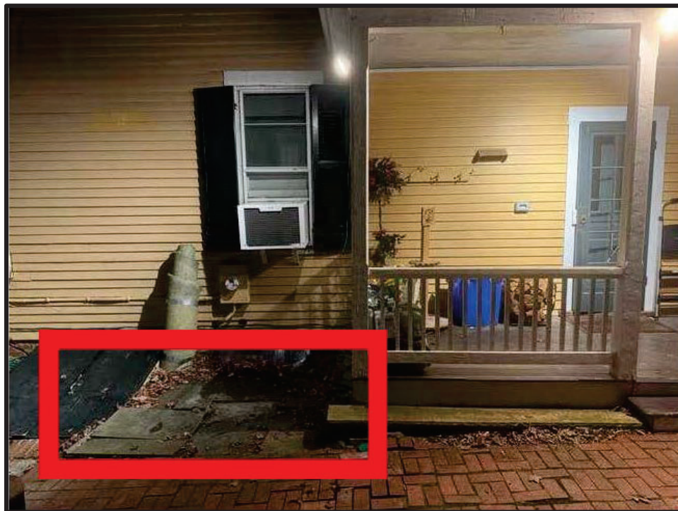
Figure 4. The applicant provided this diagram to show the location of the pad holding the heat pump and condensing unit in the rear yard.
