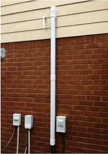
Figure 7. This representative photo provide by the applicant shows the plastic covering that will installed on the rear elevation to house the refrigerant lineset. It will be painted to match the color of the house.
