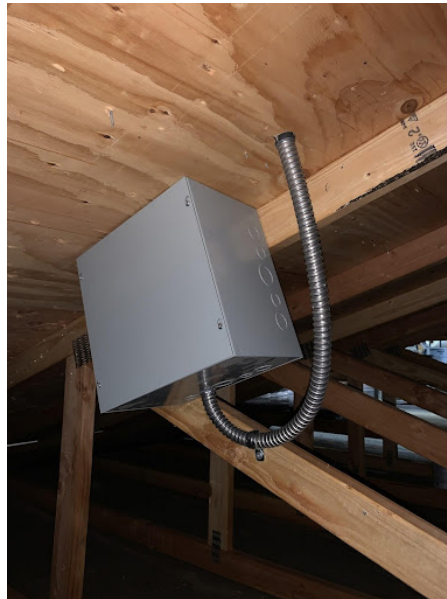
Figure 35. Conduit to Attic Enclosure
