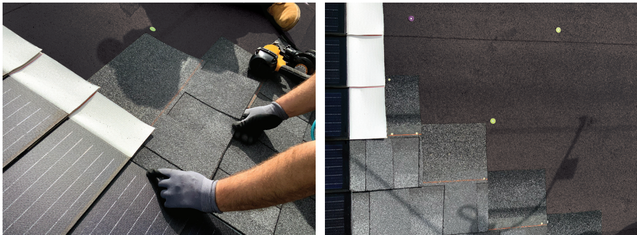
Figure 28. Shingle offsets on right edge of array
