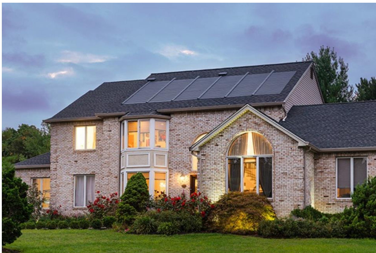
Figure 6: An installed Timberline solar shingle roof. Note: the vertical members cover the wiring to connect each shingle.
