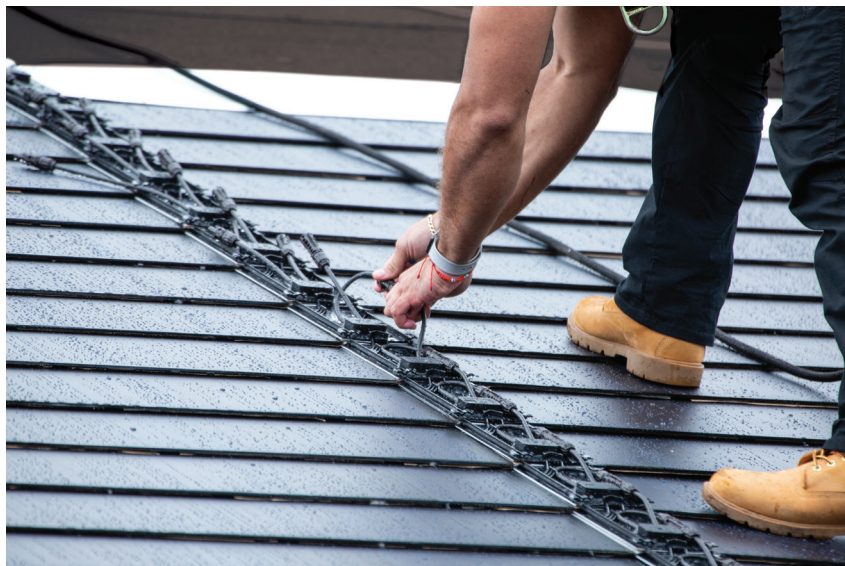
Figure 17. Ensure that vertical wire channels are straight
