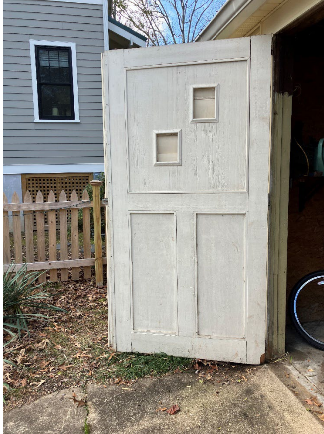
Figure 14: The applicant provided this photo of the interior of a garage door to show it is not the original
