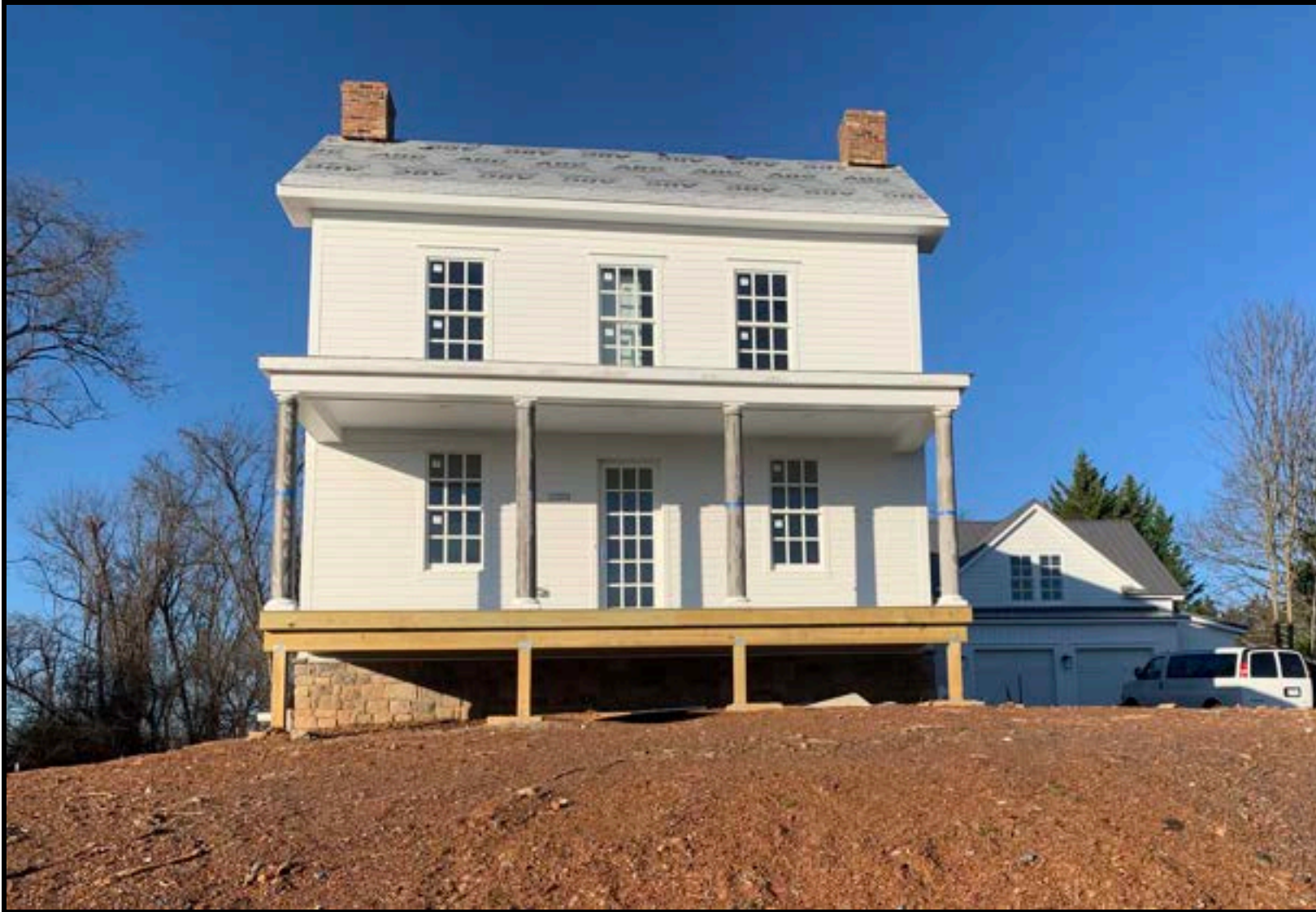
Figure 11: The front elevation on January 11, 2024. Note that fill dirt will be added to reduce the distance from the porch floor to ground to 30 inches or less so no railing is required, and the posts supporting the porch flooring will be wrapped in stone to match the foundation.
