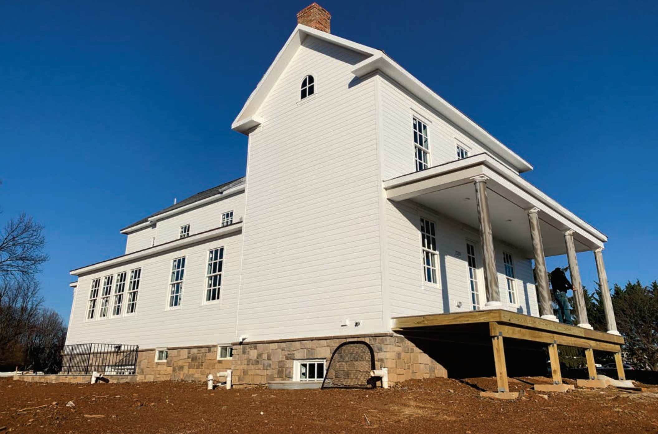
Front and Left-Side Elevations of the Cephas Summers House Chris Berger Site Visit 1.11.24
