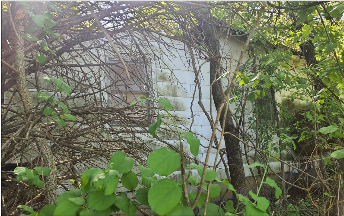
Figure 11: View of ruinous tenant building facing southwest.
