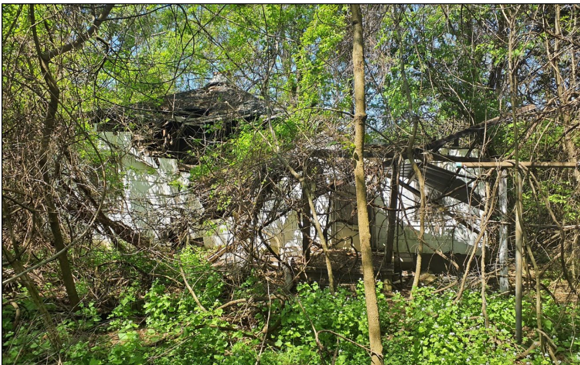
Figure 10: View of ruinous tenant building facing south.
