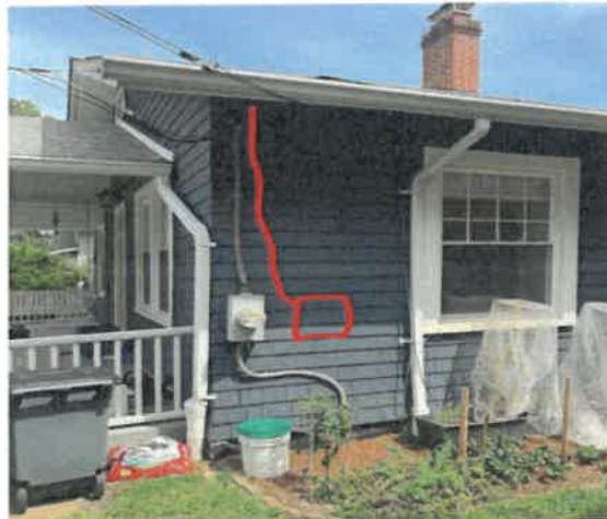
Utility Side Example After Installation
