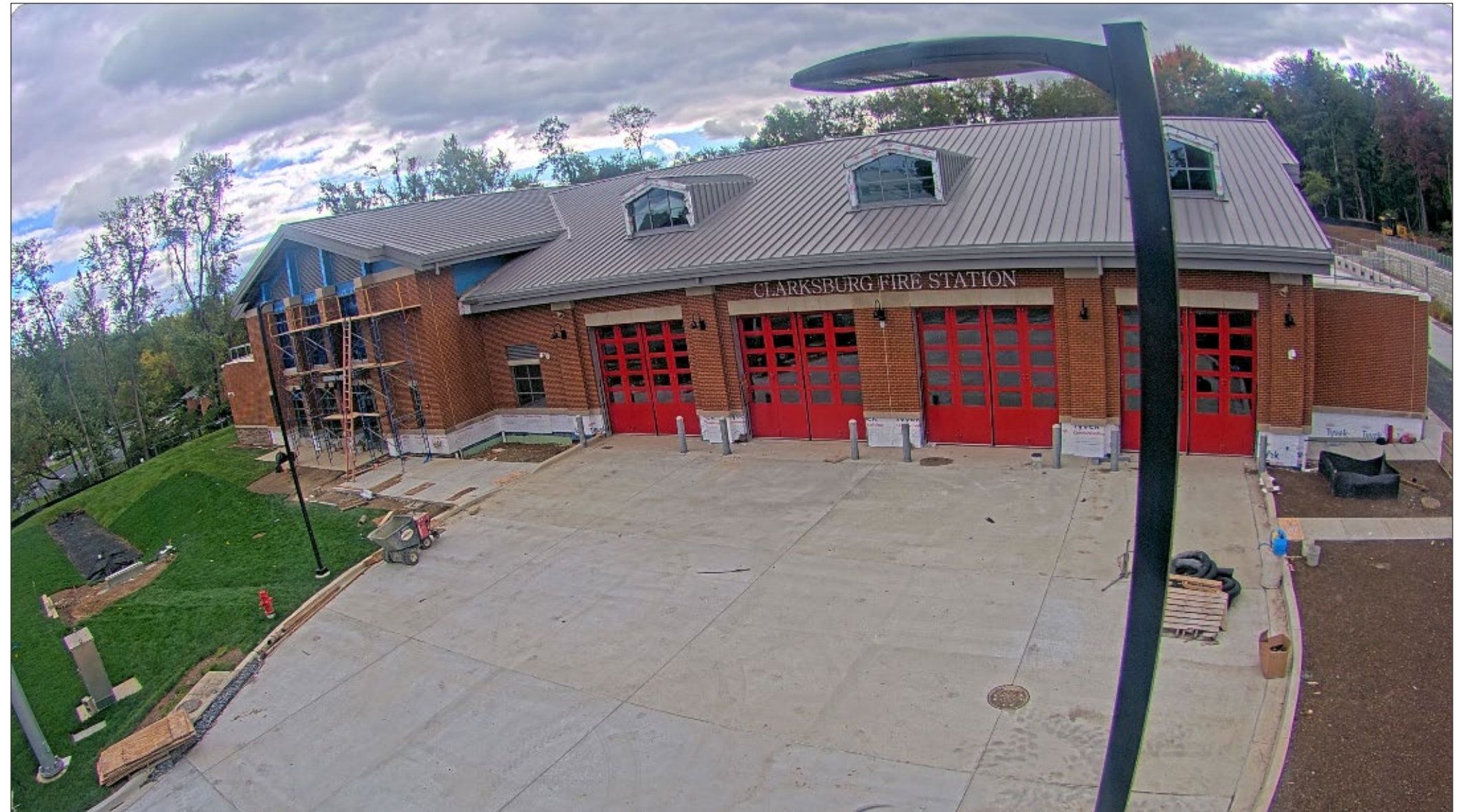
Construction progress as of October 15, 2023. Image source: Montgomery County Department of General Services
